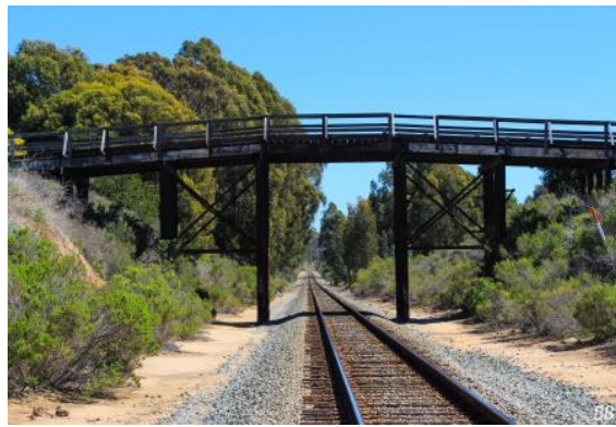
Construction of the Paradise del Mare coastal access trail may require construction of a new bridge across the UPRR as the existing bridge may not meet current standards. A new bridge may cost approximately $1.5 million.
