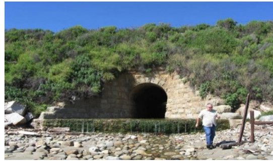
The existing UPRR Las Varas Creek Tunnel would be used to provide beach access from the one mile-long Las Varas coastal access trail. Use of this tunnel would require an easement from UPRR, permits, and possible improvements to raise the trail above stream flow.
