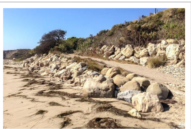
Past repairs of the Aniso Coastal Trail included installation of almost 500 feet of rock revetment to protect the trail from erosion as well as this beach access ramp. Similar improvements are needed along the currently damaged segment as the location of the UPRR precludes landward trail relocation.
