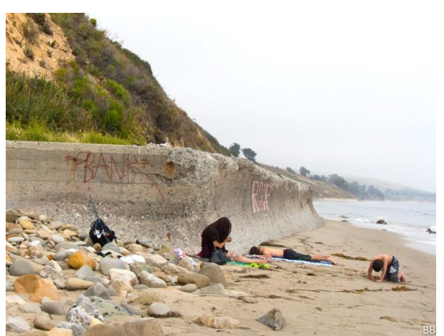
Over 1.5 miles of seawall have been constructed along the Gaviota Coast, including this 0.7-mile segment south of Arroyo Hondo. To avoid incremental armoring of other sections of Coast, the County should pursue longer-term planning, including managed retreat of UPRR and US 101 (as needed).
