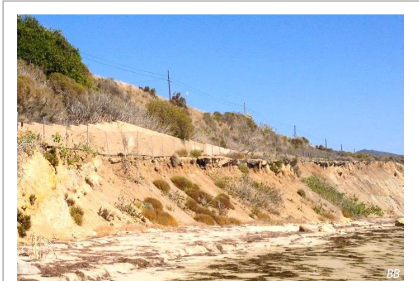
The 580 foot-long damaged segment of the Aniso Coastal Trail is being undercut by erosion and may be destroyed by major winter storms. This segment lacks rock revetment that have successfully protected two other segments of this trail.
