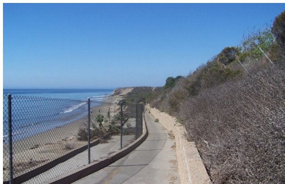
Repair of the 580 feet of damaged El Capitan to Refugio coastal trail would restore and enhance public access to this highly scenic coastline. The UPRR (right) prevents trail landward relocation.
