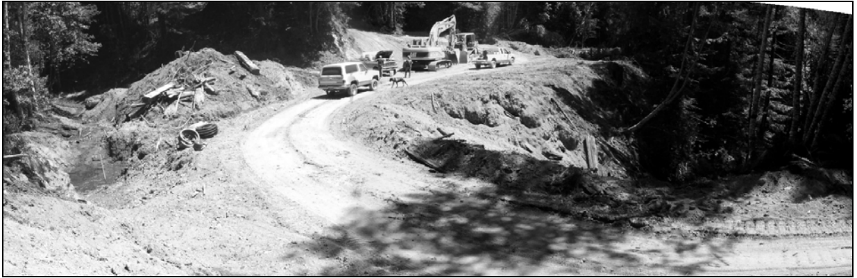
Figure X-D-18. Site #3, 1311 Road, before excavation. This is a 3 shot panoramic compilation photo taken from the cutbank on the right approach to this Humboldt stream crossing. The site has been brushed out and a temporary flex pipe has been installed along the right hinge line to divert active flow around the work area.
