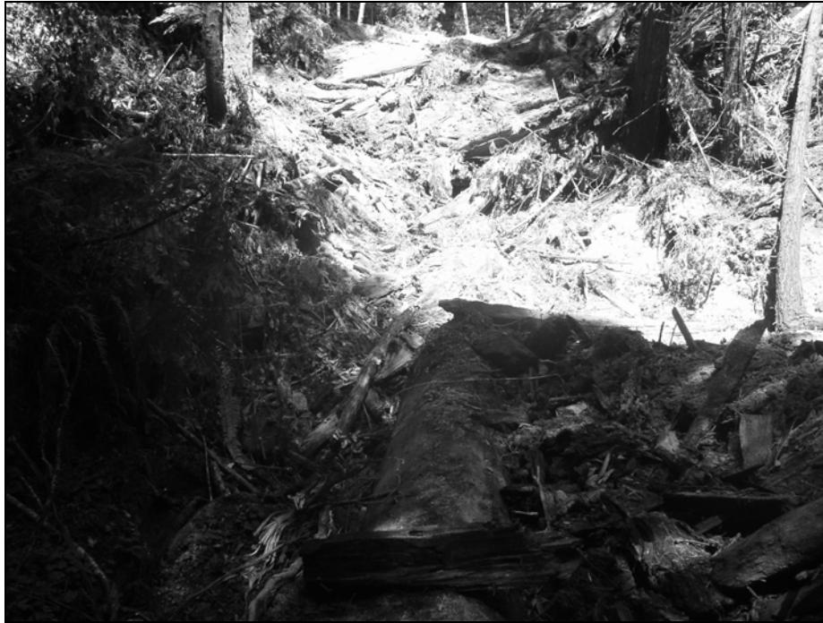
Figure X-D-20. Site # 3, 1311 Road, during excavation. This picture was taken near the Bot of the stream crossing. The picture view is looking upstream with the outboard edge of the road in the upper center portion of the photo. Some fill has been excavated from the outboard edge of the road downslope towards the Bot and a swath of brush as been cleared to the Bot, in preparation for continued excavation.
