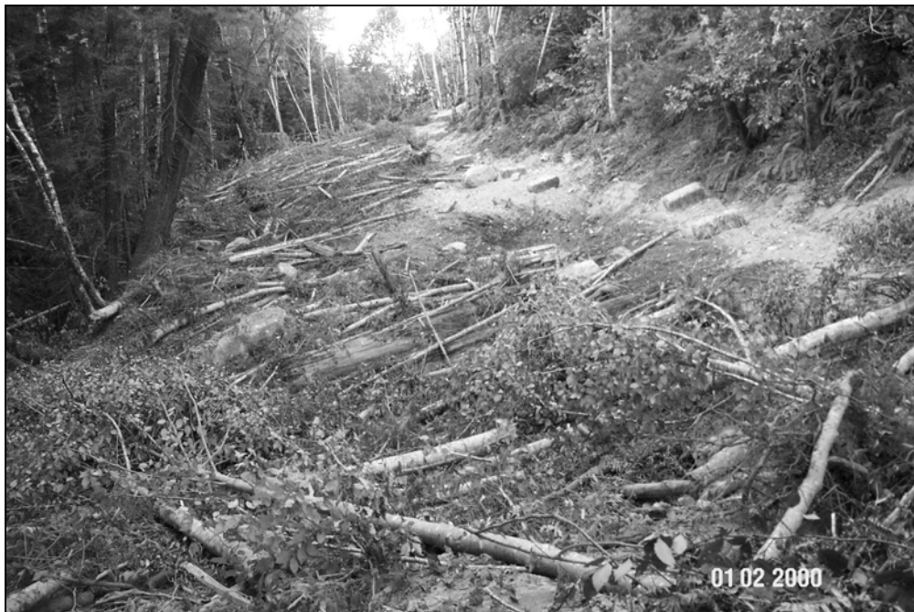
Figure X-D-27. Site # 2, 1312 Lower Road, after excavation. This picture was taken from the same viewpoint as above. The unstable road fill has been completely excavated. Straw mulch and seed had not yet been spread in this picture (note straw bales near former cutbank).
