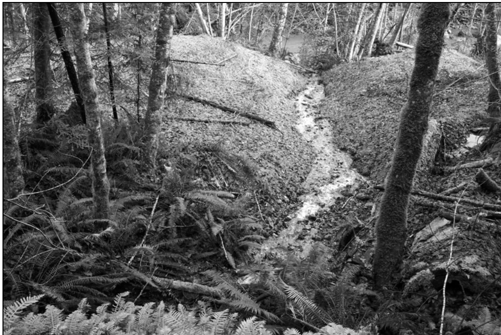
Figure X-D-15. Site # 11, 1305 Road, after excavation. This picture was taken from the same viewpoint as above (Figure X-D-13 and Figure X-D-14) during a heavy rainfall event. Note the stream channel bed has developed a self armoring “lag” deposit during the first season’s rainfall. Redwood Creek is in the background.
