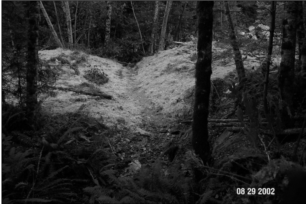
Figure X-D-14. Site #11, 1305 Road, after excavation. This picture was taken from the same viewpoint as X-D-13. The stream crossing has been excavated, mulched and seeded. See same view below after heavy rainfall (Figure X-D-15).
