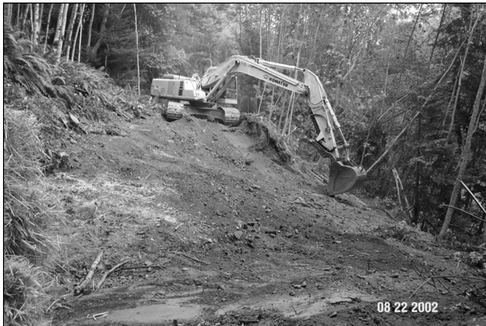
Figure X-D-11. Site #10, 1305 Road, during excavation. A potential road fill landslide was excavated at this site. Unstable outboard road fill was excavated and endhauled to a stable storage location, creating an outsloped road surface (see Figure X-D-12).
