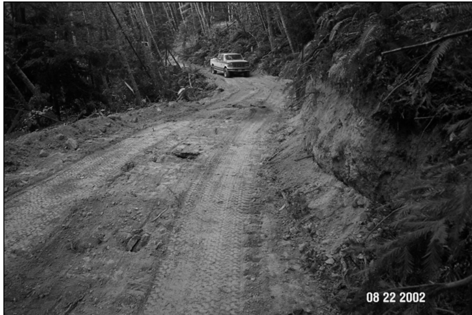
Figure X-D-16. Site # 13, 1305 Road, before excavation. A potential road fill landslide was excavated at this site. Unstable outboard fill was excavated and endhauling to a stable storage location, creating an outsloped road surface (see Figure X-D-17).
