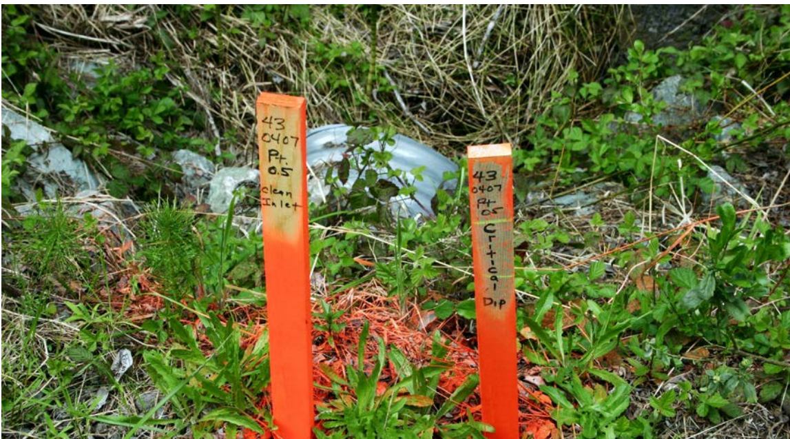
FIGURE 236. For large landowners, maintenance tasks can be identified on a data form, and staked on the ground by inventory crews. This small stream crossing needs a critical dip to prevent future stream diversion, and the inlet needs cleaning; tasks to be completed by maintenance crews or contractors.
