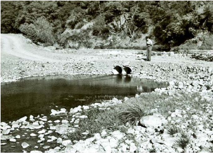
FIGURE 127A. Summer low-water crossing of a Class I (fish-bearing) perennial river. Coarse, clean streambed material has been used to ramp up and over the flowing water. Two embedded culverts have been installed at water level to allow for uninterrupted flow and the migration of young fish.
