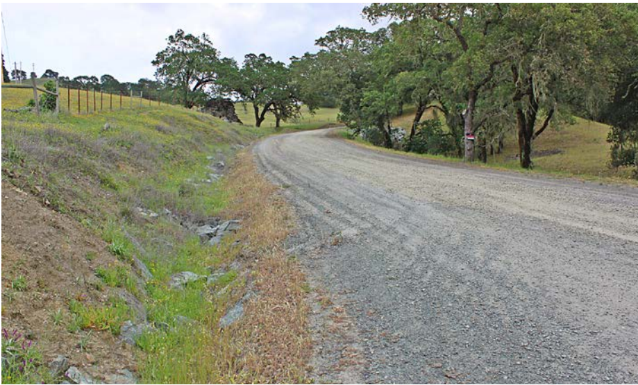
FIGURE 246B. The road was upgraded by crowning and additional ditch relief culverts were installed to disperse ditch flow. The pasture was also fenced to keep cattle off the erodible sideslopes.
