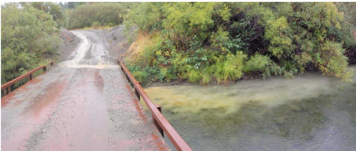
FIGURE 21. Road approaches to bridges are often hydrologically connected. This through cut approach to a temporary bridge drains directly into the stream.
