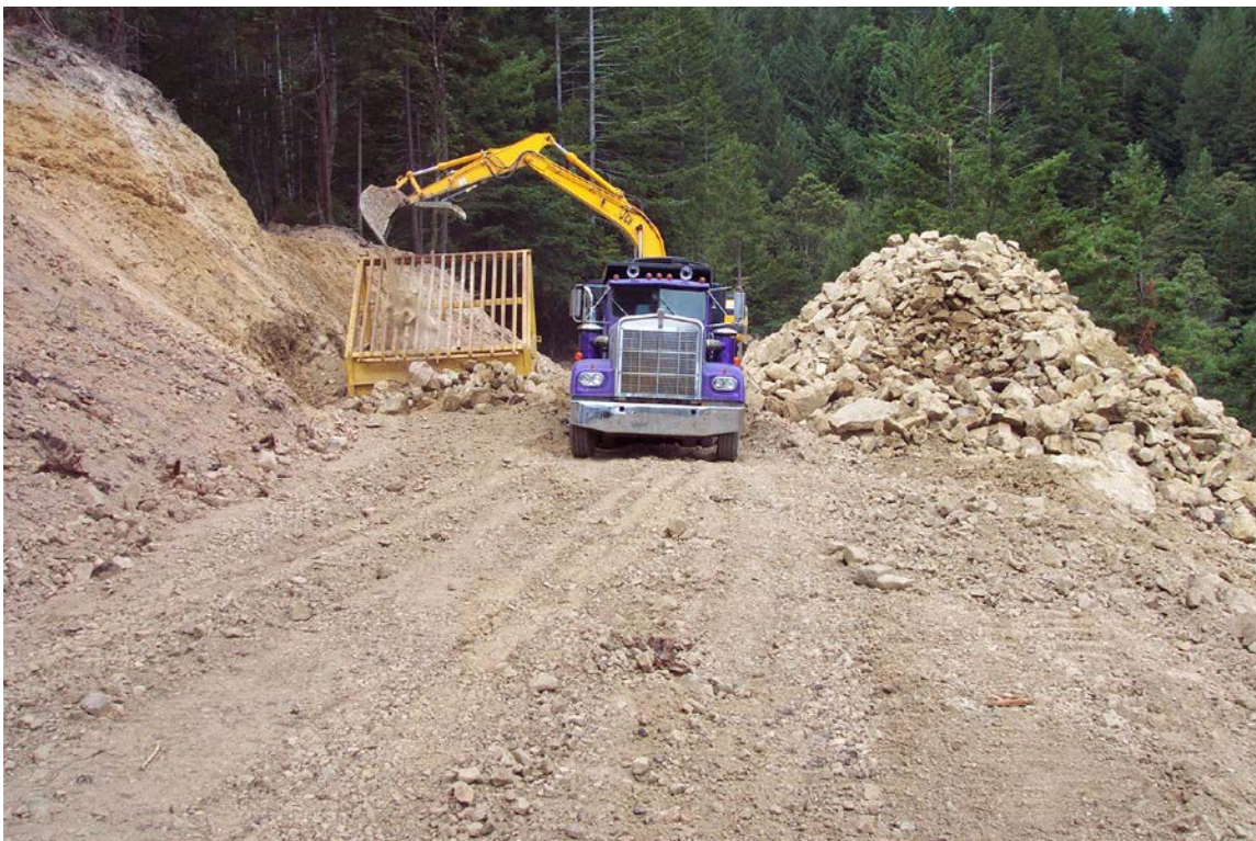
FIGURE 60. This rock pit is easily worked by an excavator, but the material contains abundant fine grained particles. Here, a Grizzly rock screen is used to separate high quality rock armor from fine grained waste materials. As in this photo, waste materials should be endhauled to a stable spoil disposal site rather than sidecasting onto steep, unstable or streamside slopes.
