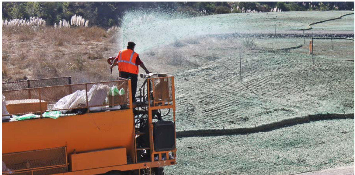
FIGURE 288. Hydroseeding (spraying a slurry of water, mulch, seed and fertilizer) on bare soil areas can be an effective erosion control and revegetation treatment for large disturbed areas, or for bare soil areas along open roads. It is most useful for treating spoil disposal sites, after they have been graded and smoothed, and for treatments along newly upgraded roads where the truck or trailer can have easy access. Hydroseeding decommissioned roads is more difficult because access is cut off as the treatments progress. Rather, hand seeding and mulching is usually the preferred treatment.
