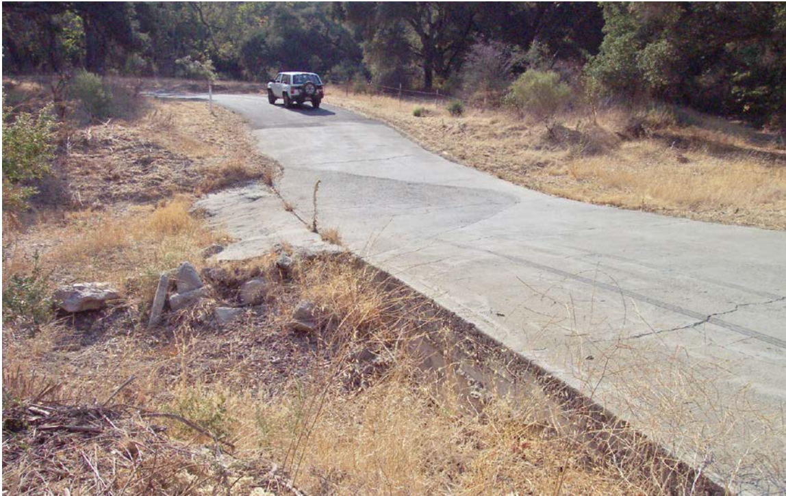
FIGURE 123. Flow in this hardened ford is from right to left. Low flow energy dissipation has been built into the center of the structure, but high flood flows have scoured to the base of the concrete ford in the foreground. Both the hardened ford and the downstream energy dissipation must be broad enough to encompass and contain the expected 100-year design flood flow.
