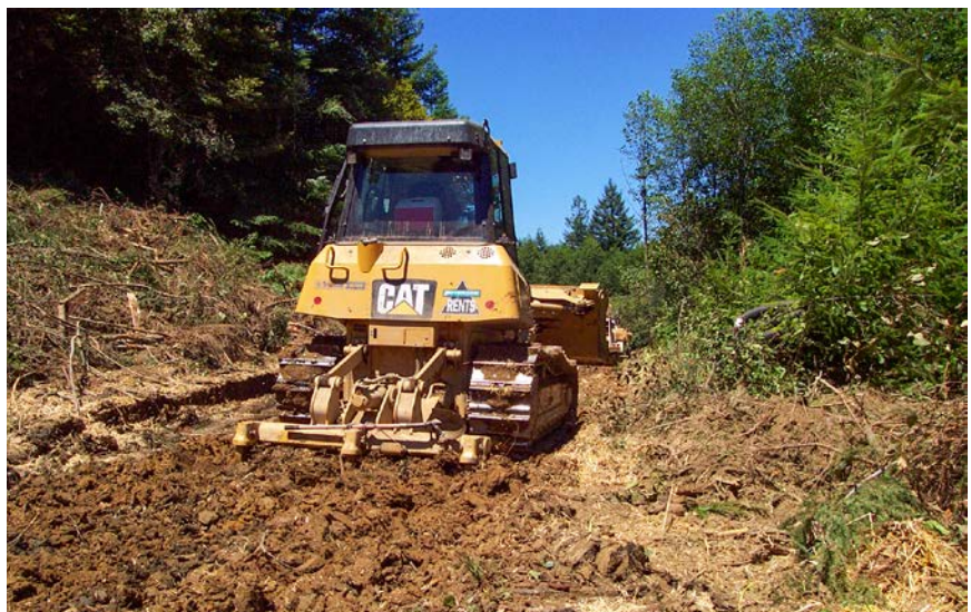
FIGURE 283. Small bulldozer with hydraulically operated rippers (three 30 inch long steel chisels) is decompacting a seasonal road as a part of road decommissioning. Road ripping should be a standard decommissioning practice. All decommissioned roads should be ripped to decompact the road bench, improve and speed revegetation and reduce surface runoff. If the road is to be outsloped, and spoil is placed on the former roadbed, the compacted road bench should first be ripped to a depth of 18 to 24 inches, or greater. If it isn't ripped, infiltrating water will pond on the compacted surface and may cause soil saturation or contribute to slope failure.
