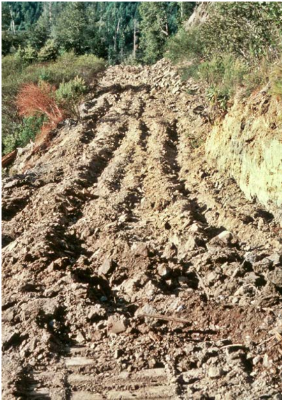
FIGURE 290. Deep, thorough ripping is a good treatment to largely eliminate surface runoff and “hydrologically disconnect” a former road from nearby stream channels.
