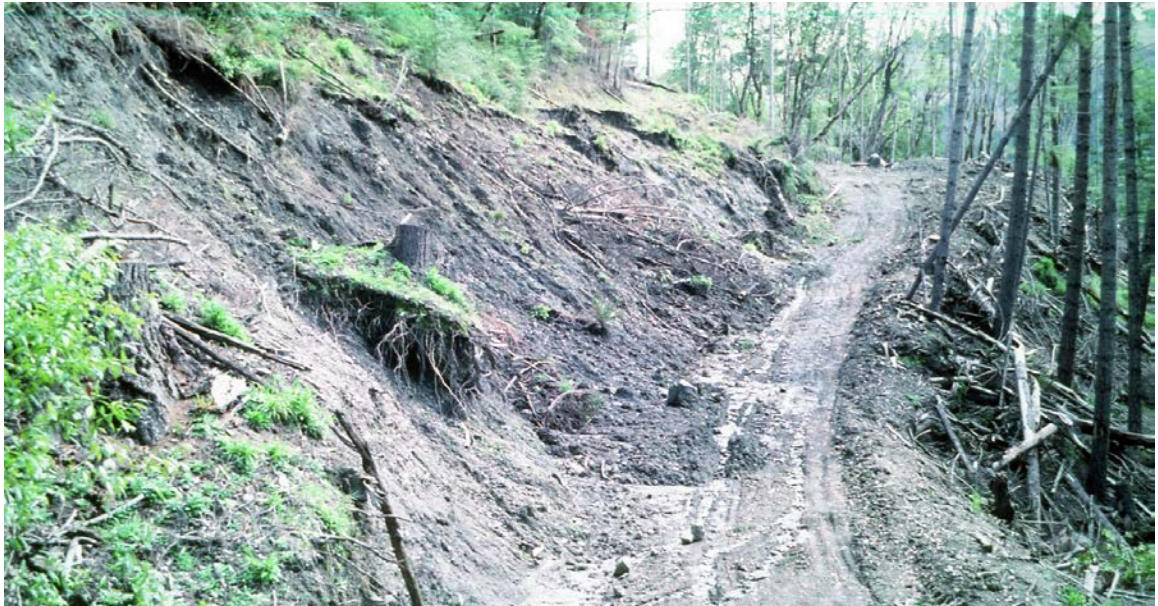
FIGURE 56. This forest road was constructed through wet, unstable soils and subsequently experienced shallow slope failures and rapid erosion rates for a number of years following road building.
