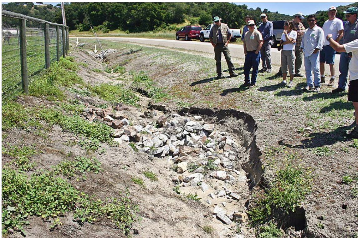
FIGURE 183. Poorly installed rock check dams installed in a rural roadside ditch to control erosion. The rock dams were spaced too far apart (see arrows farther up the ditch for nearby dams) so that erosion between the dams led to downcutting and undermining of upstream structures. The dam in the foreground failed because 1) it was not keyed into the side walls or channel bed, 2) the spillway capacity was insufficient, and 3) there was no energy dissipation at its base.
