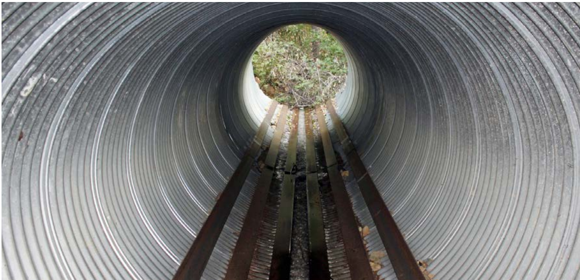
FIGURE 89. Steel plates have been welded onto the lower 25% of the invert of this 6 ft diameter galvanized culvert. The steel provides protection against abrasion by coarse bedload transport.
