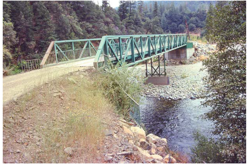
FIGURE 119. It is important that all bridges used to transport vehicles and equipment be properly designed or evaluated by a structural engineer before they are put into use. This long, truss-reinforced bridge was fabricated from two 90-foot long railroad flatcars with a center pier support that can be folded up under the bridge during winter flood flows. The center pier must be put down to haul heavy loads across the bridge.
