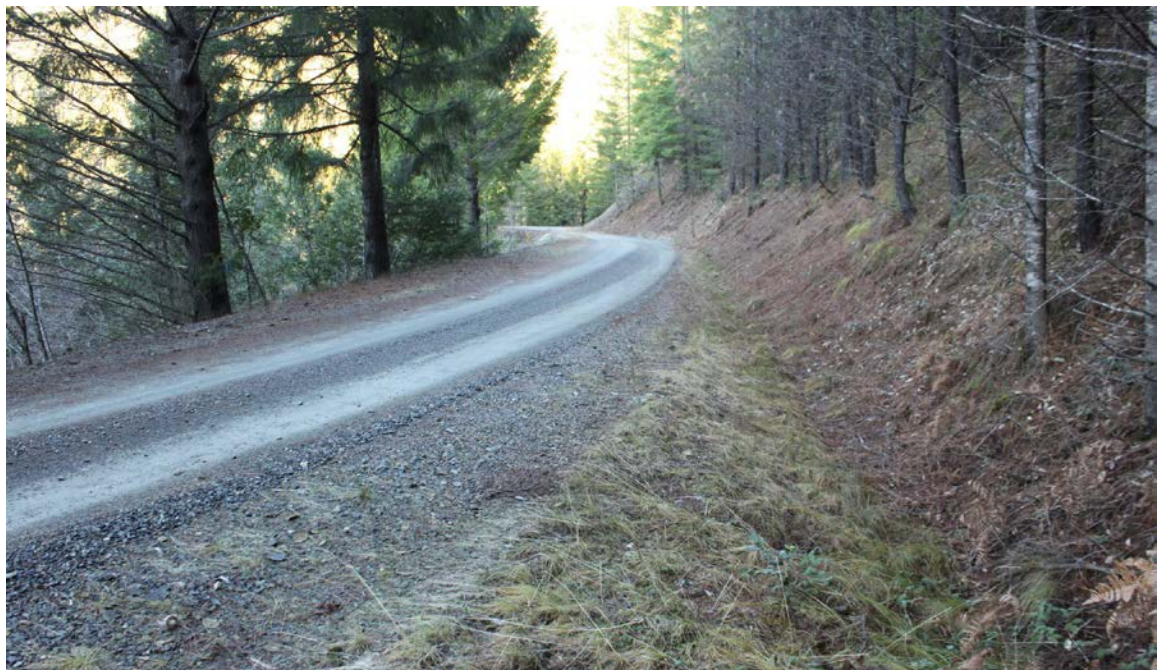
FIGURE 44. This insloped, gravel surfaced road drains to a vegetated ditch. The ditch is connected to a stream crossing culvert, but the heavy vegetation in the ditch prevents sediment from being delivered to the stream.
