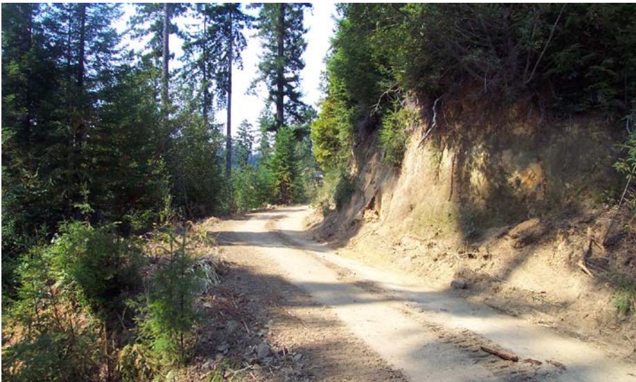
FIGURE 270A. Tall, dry cutbank where the road cut across the nose of a ridge. Just down the road an unstable fill was excavated to prevent a potential fill slope failure and this favorable site was used for spoil disposal.
