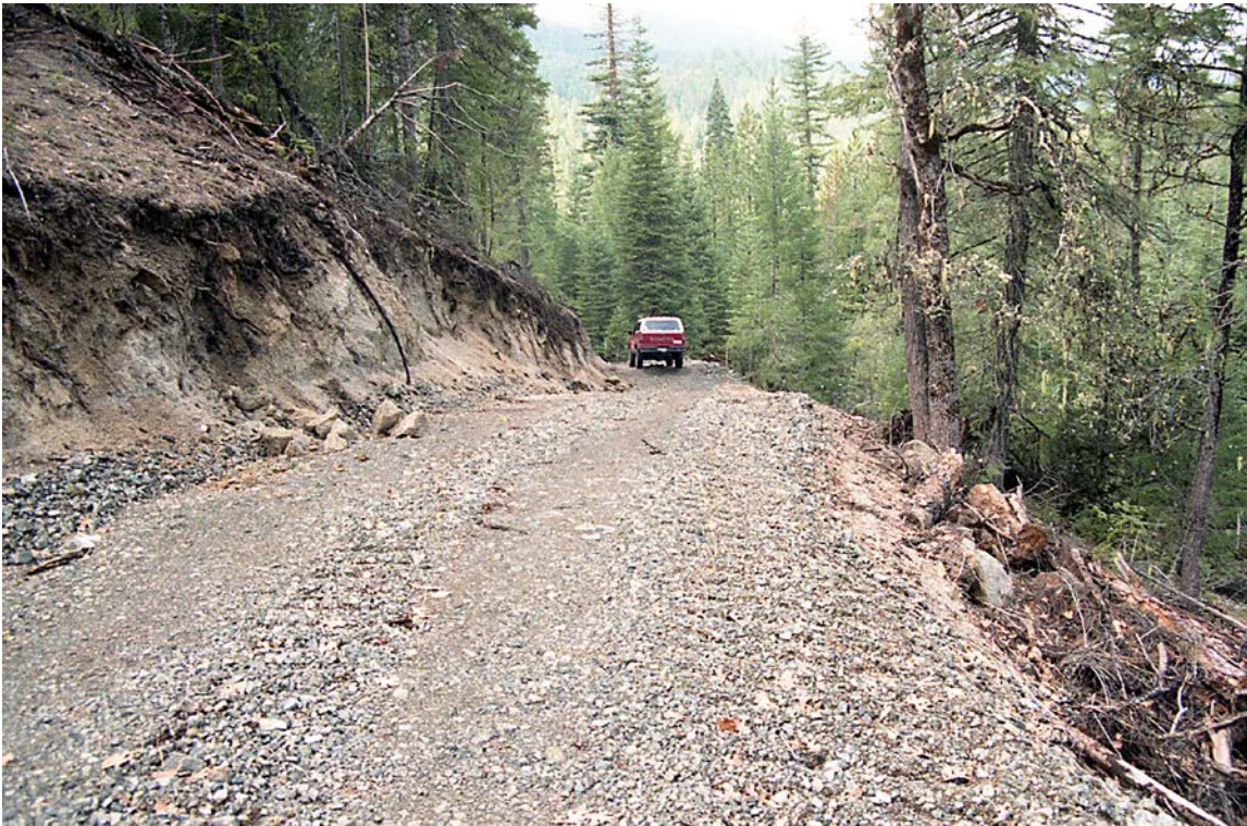
FIGURE 172. Newly constructed, outsloped forest road with accumulated line of slash, called a filter windrow, at the base of the fill to catch soil eroded from the new fill slope. Slash should be placed at the base of the fill, and not incorporated into the soil material. Filter windrows are most important to install where roads approach and cross stream channels. This outsloped road conforms to the topography of the land and incorporates rolling dips at natural swales to shed surface runoff.
