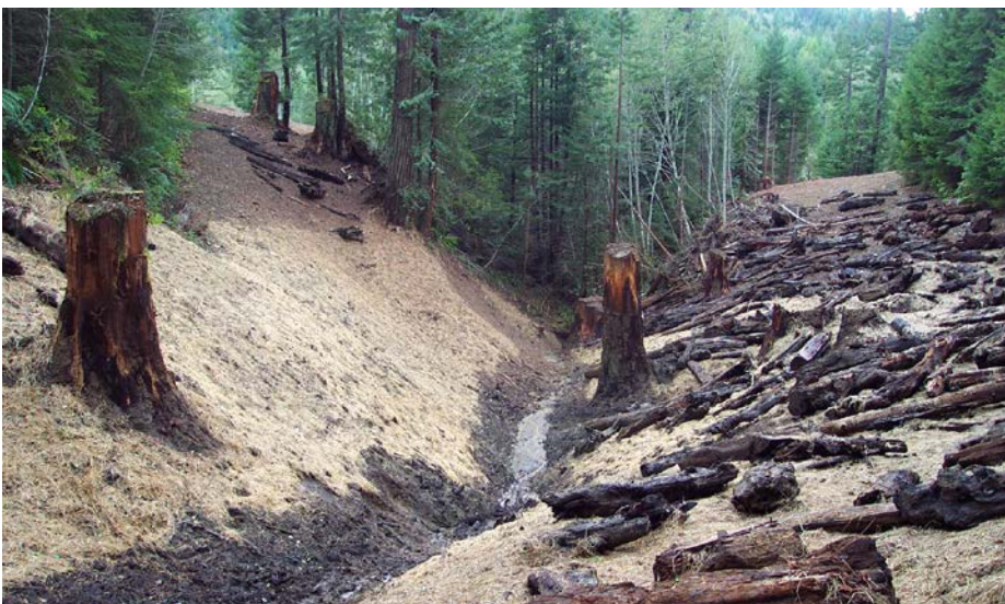
FIGURE 266C. The channel was excavated (exhumed), and the side-slopes were sloped back to stable angles, exposing several buried stumps that signaled the level of the original ground surface. The bare slopes were then seeded, mulched with straw, and planted with trees. All the logs visible on the right bank had been buried in the crossing fill. They were removed and placed on the final ground surface.
