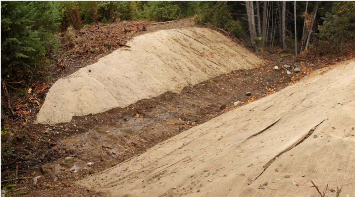
FIGURE 287. Most often, a uniform cover of straw mulch is all that is needed to temporarily control surface erosion on the excavated sideslopes of decommissioned stream crossings until they can naturally revegetate. Wood chips, or native brush and slash, also work well to control surface erosion in some environments. Here, jute netting has been used instead of straw, as a trial treatment. Rolled and tacked erosion control blankets, or jute netting tacked over a layer of straw mulch, can be used on sideslopes that are steeper than about 2:1 (50%). To avoid spreading non-native weed species, many areas can employ rice straw whose seed and weed species are not adapted to growing in most upland environments. Rice straw mulch also has a roughness or “stickiness” that allows it to hold in place on slopes steeper than wheat or grass straw.
