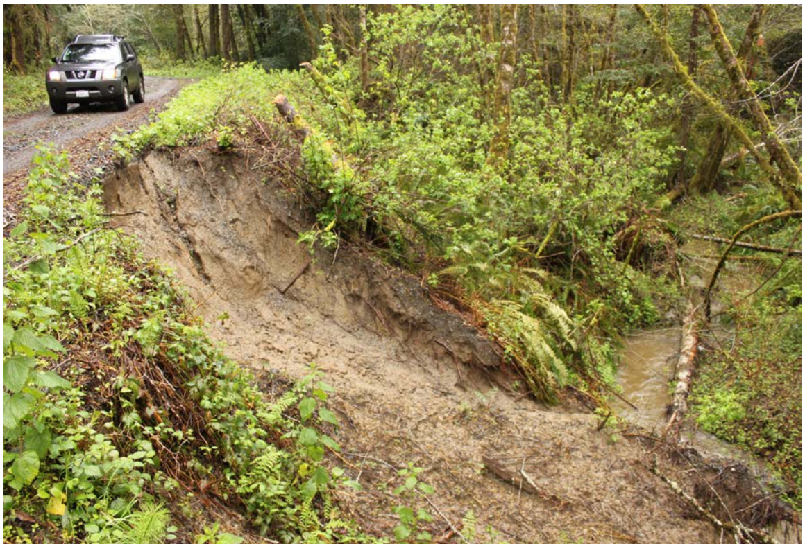
FIGURE 4B. At a smaller and more common scale, fill slope failures on roads built on steep slopes near stream channels have a high likelihood of delivering sediment directly to the stream channel.
