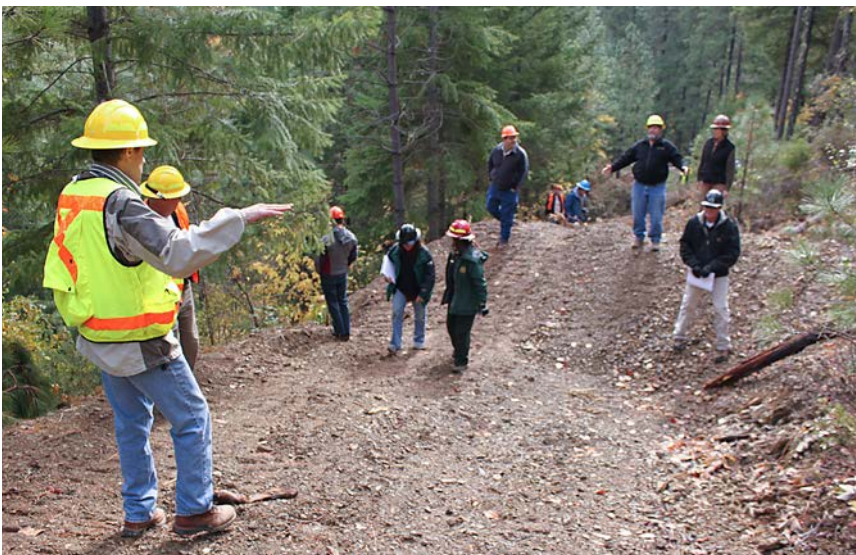
FIGURE 281. Between treated stream crossings and fill slope excavations, decommissioned roads should have permanent road drainage treatments, including road decompaction (ripping or subsoiling) and constructed cross road drains. Cross road drains are permanent road drainage features, like waterbars but much more substantial so they will function indefinitely and will not be broken down by rainfall, runoff or any kind of unwanted recreational traffic (usually bicycles or motorcycles). Like waterbars, they are usually excavated into the firm roadbed, mounded on the downhill side and spaced closely enough to prevent significant erosion on the roadbed or below the point of discharge.
