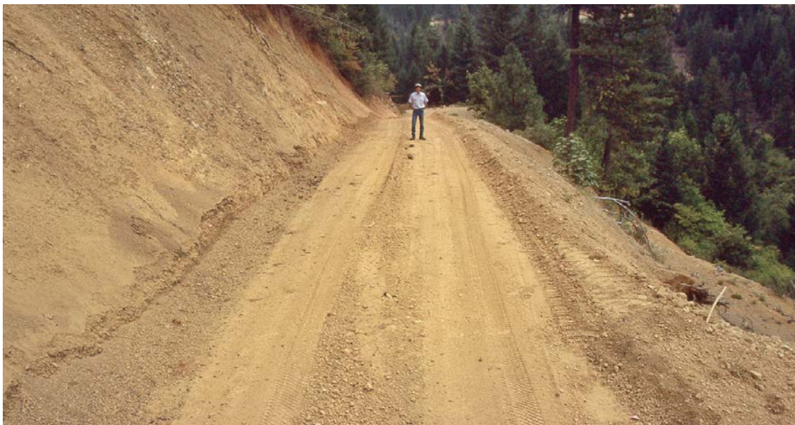
FIGURE 42. Short road reach where a soil berm has been intentionally constructed along the outside edge of the road prism to prevent surface runoff from flowing over the highly erodible fill. To prevent the accumulation of too much runoff, the berm can be intermittently breached and a small flared inlet and culvert or sheet metal berm-drain installed to carry runoff downslope past the base of the erodible fill slope.
