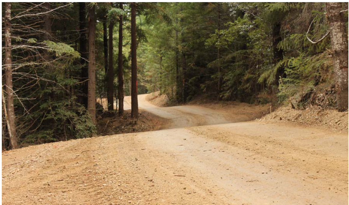
FIGURE 28. Well built, outsloped road displaying minimum cut, smooth free draining surface, and no outside berm. The road contours the topography and its rolling grade and rolling dips disperse surface runoff.
