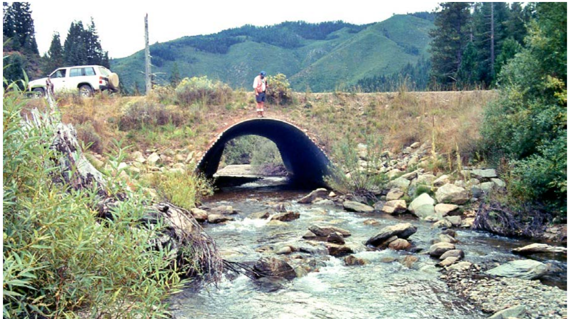
FIGURE 72. This bottomless plate arch was installed to provide fish access through the stream crossing. Each abutment is comprised of a concrete foundation and the stable stream-bed ensures continuous aquatic passage.
