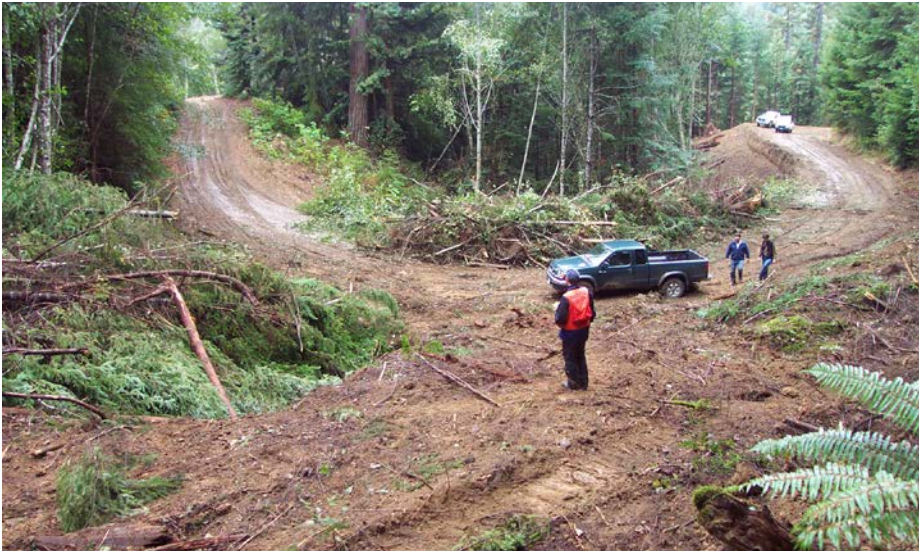
FIGURES 266A–E. This five-photo sequence shows the permanent decommissioning of a stream crossing on a former logging road. The road was no longer needed and has been permanently closed. The first step (266a) was to clear vegetation from the fill and from upstream of the crossing, where the channel had been filled with logging debris several decades earlier.
