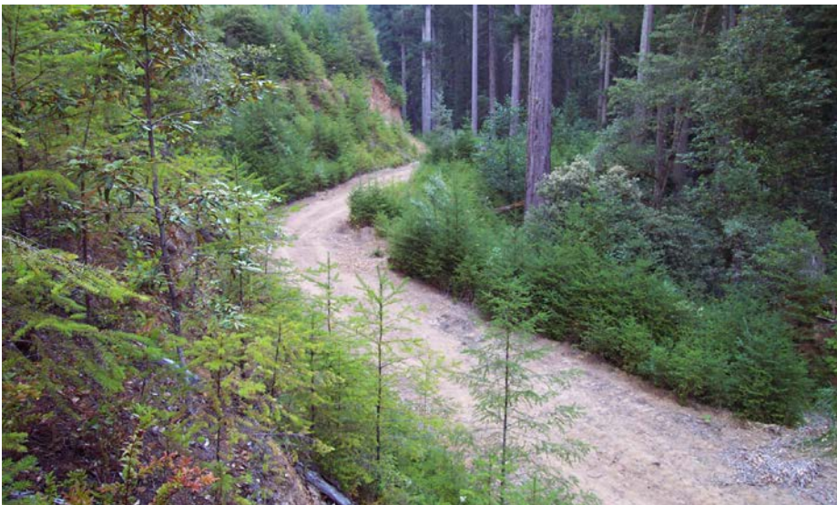
FIGURE 274A. Abandoned forest road that was reopened for decommissioning and erosion prevention treatments. The proposed treatment was to completely restore and recontour the hillslope in this biological reserve and conservation area.
