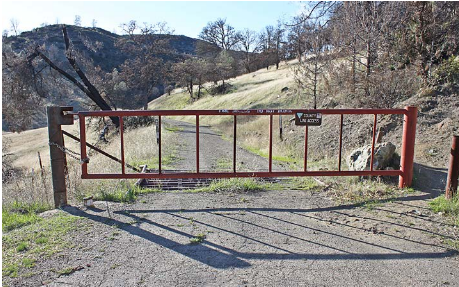
FIGURE 249A. There are a variety of ways to close a road to off-season traffic, but it should always be remembered that barricading the road does not by itself prevent erosion along the alignment. Gating closes the road to unauthorized traffic but still allows for winter maintenance and inspections.
