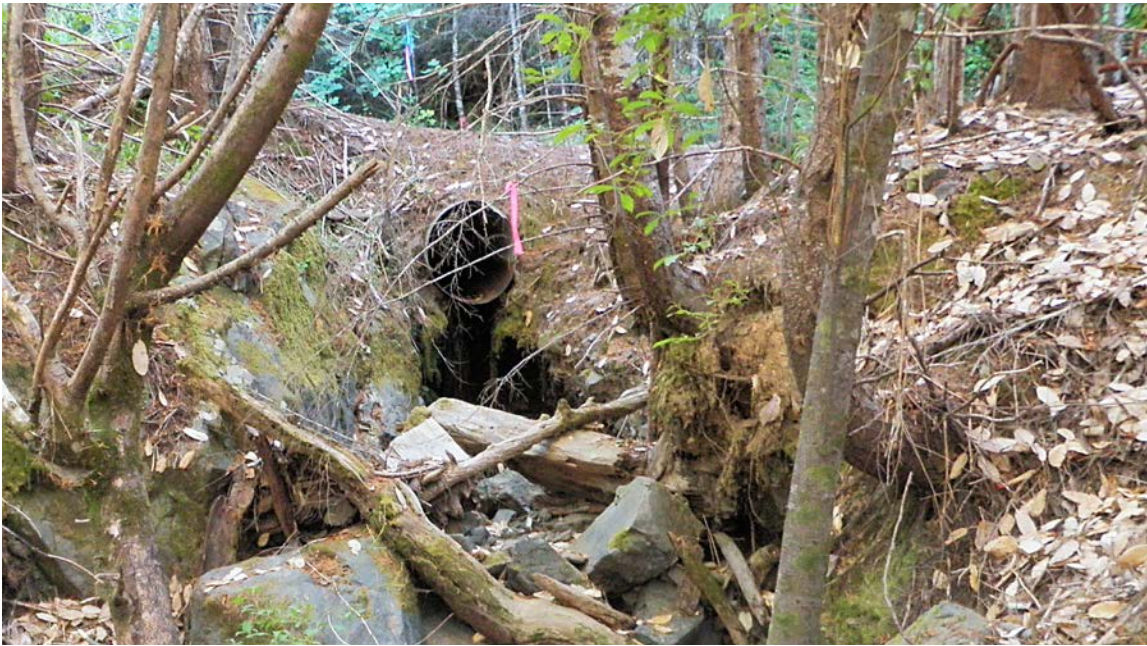
FIGURE 217A. Culverted stream crossing on a permanent forest road before upgrading to the 100-year design standard (including debris and sediment). The before and after photos of the culvert outlet are taken from the same location.
