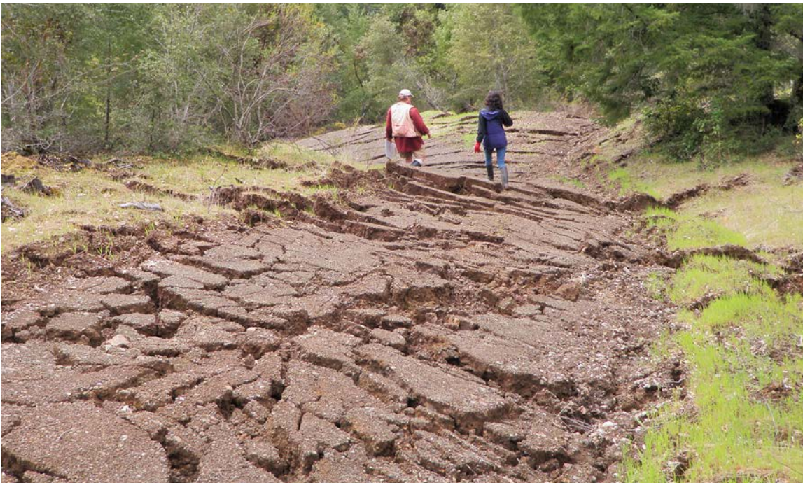
FIGURE 206. This rural road traversed a large unstable hillslope that showed widespread movement during an exceptionally wet winter. The road did not cause the instability but it is no longer useable. Alternative access should be developed wherever roads cross highly unstable terrain. This road should be decommissioned so no additional erosion and instability is caused by the road and its drainage structures.
