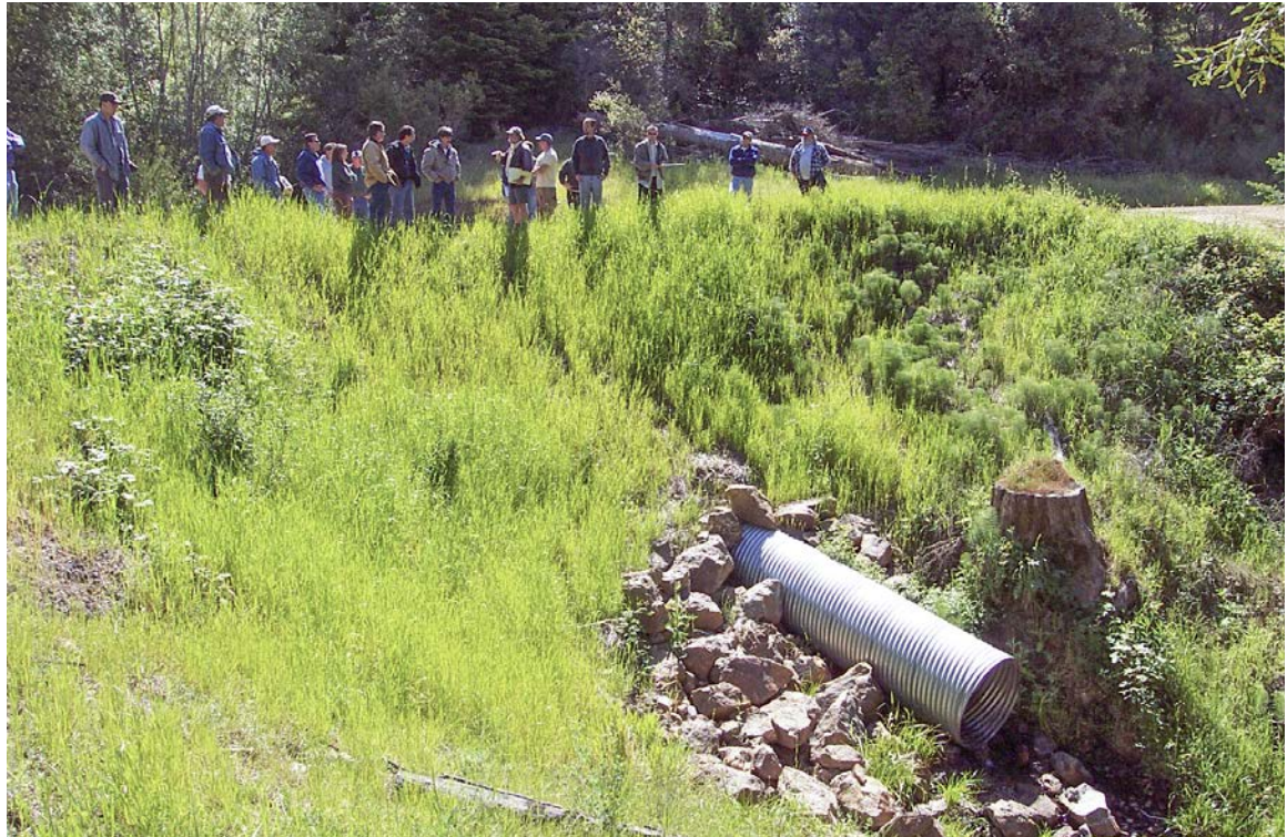
FIGURE 80. Rock armor placed around this culvert where it emerges from the fill slope was used to protect the stream from unexpected erosion of the new, erodible fill slope until it stabilized with vegetation.
