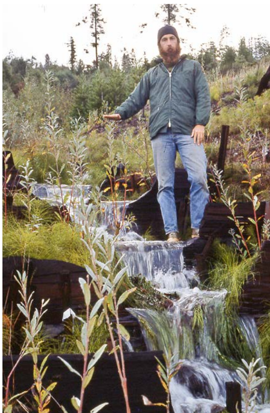
FIGURE 180. Board check dams constructed in a gully to prevent downcutting and stabilize the bed and banks. Willow cuttings planted and growing in the bed and banks will eventually stabilize the gully once their roots are well developed.
