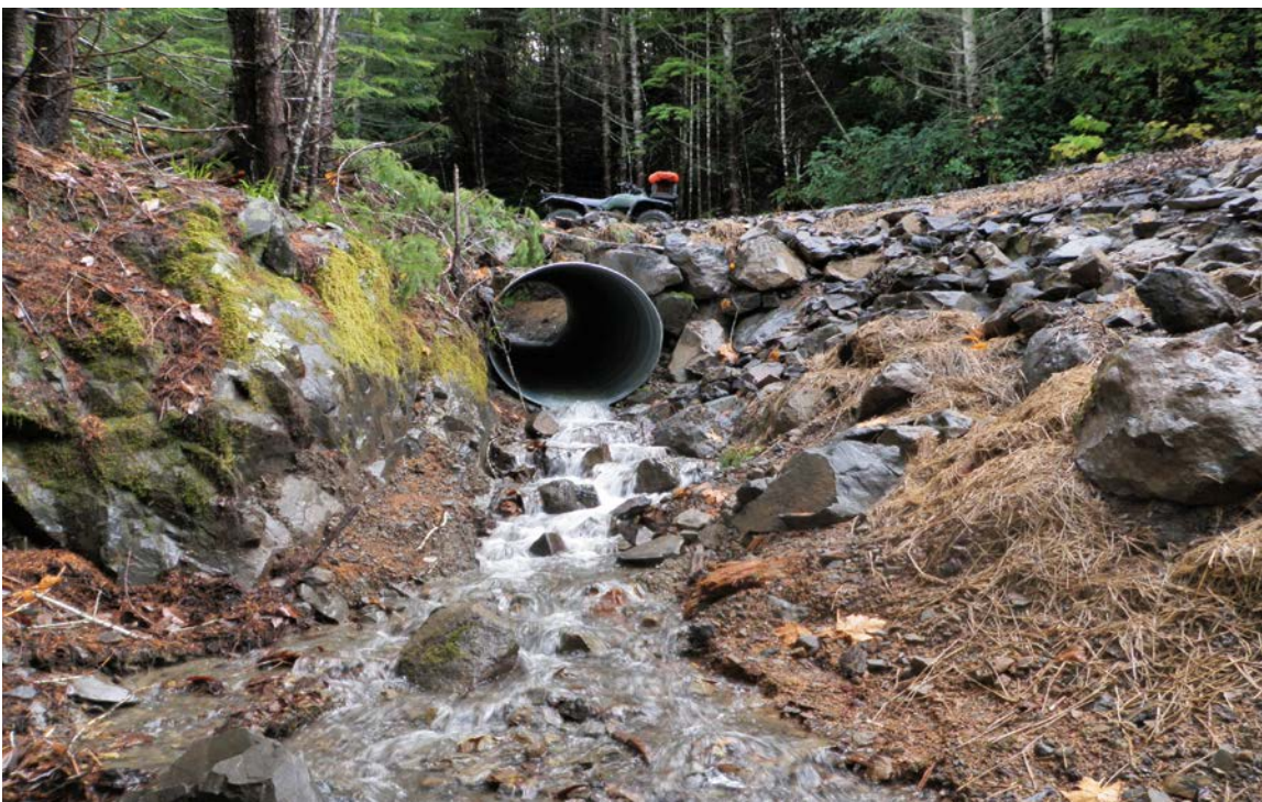
FIGURE 217B. The same stream crossing after culvert upgrading. The culvert has been set in the original streambed and the fill dipped to prevent stream diversion.
