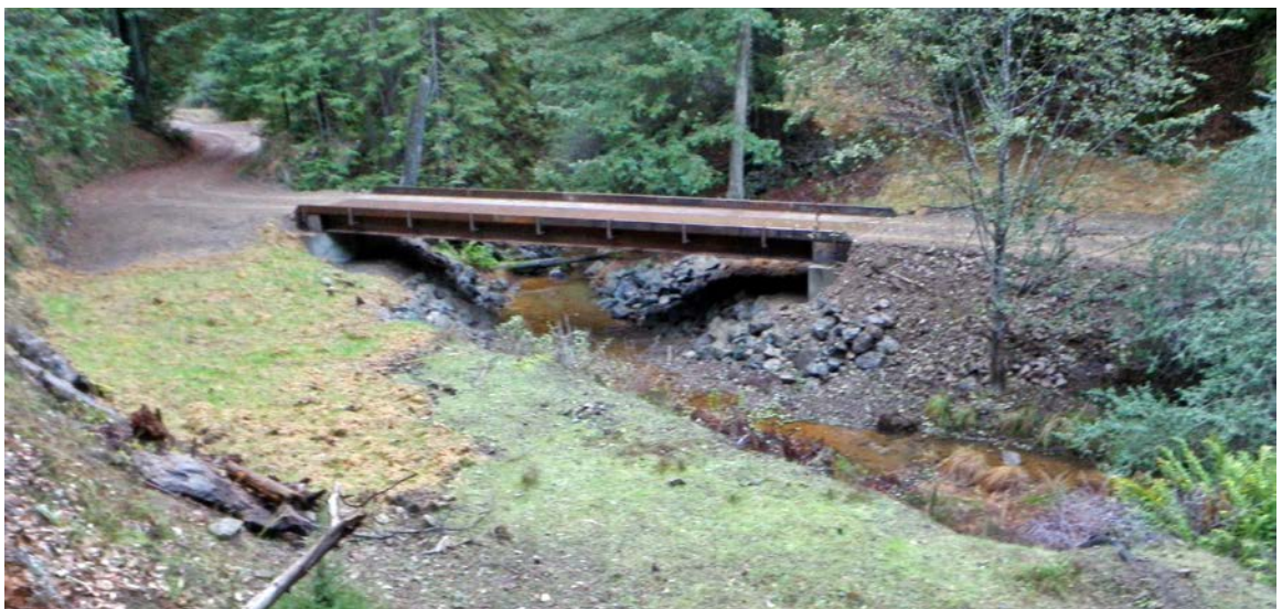
FIGURE 218B. The culverted stream crossing was upgraded to a steel I-beam and plate metal bridge to provide for passage of adult and juvenile fish. Note the concrete abutments, armored fill slope and naturally wide channel bottom through the crossing after bridge installation.
