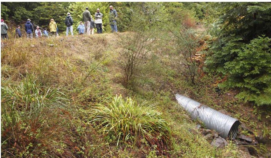
FIGURE 76. This newly upgraded 36-inch diameter culvert was installed in-line with the natural channel and at the base of the road fill. The road fill was graded to slightly less than 2:1 (50% slope) that was easily and rapidly revegetated. The culvert outlet extends at least 6 feet beyond the fill and discharges into the natural channel bed.
