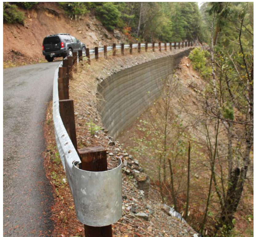
FIGURE 212. Engineered fill constructed where a fill slope failure had removed the entire roadbed.
