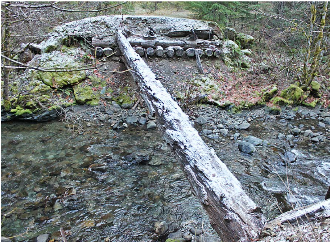
FIGURE 257. Former log stringer bridge across a large fish bearing stream has been removed, with only a single log for left foot traffic. The bridge provided the only access to over two miles of forest road containing numerous culverted stream crossings that can no longer be maintained. Roads that have not been properly decommissioned require inspection and maintenance. The roads on the other side of this bridge have recently been scheduled for decommissioning.
