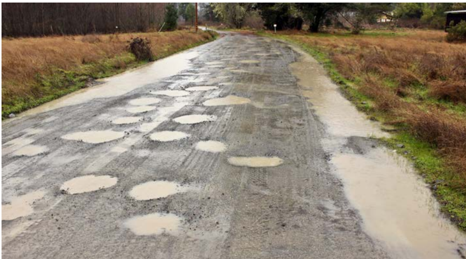
FIGURE 240. Slightly through cut, flat road exhibiting poor road drainage. Flat roads, with no gradient along or across the road, do not drain effectively and will develop potholes and mud puddles from continued traffic. Vehicles passing through standing water splashes the water and fine sediment from each hole or depression, gradually enlarging their size and depth. The through cut on this road developed by annual maintenance grading and the consequent gradual lowering of the road surface. Poor surface drainage will not improve until the road is raised and crowned, or paved.
