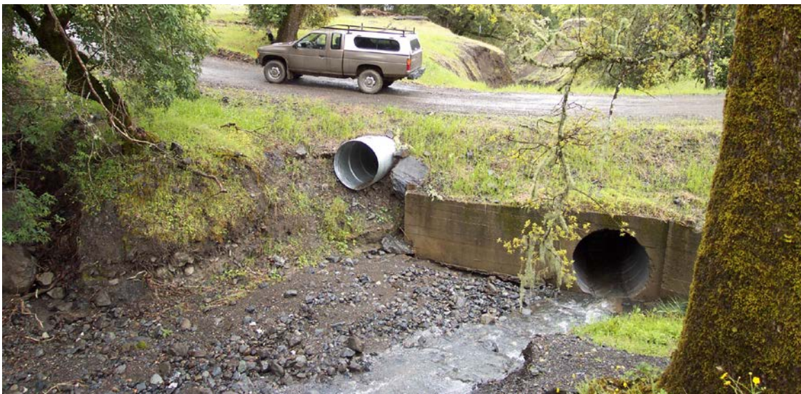
FIGURE 115. Where stream crossing culverts may not be adequately sized for the design flood flow, and they are not scheduled for immediate replacement, they can be fitted with more efficient entrances (such as the headwall seen here) as well as emergency overflow pipes installed higher in the fill. The overflow pipe provides relief during the large flow events or when the main culvert becomes plugged with debris. This overflow culvert experienced flood flow during the first winter after it was installed (See Figure 111).
