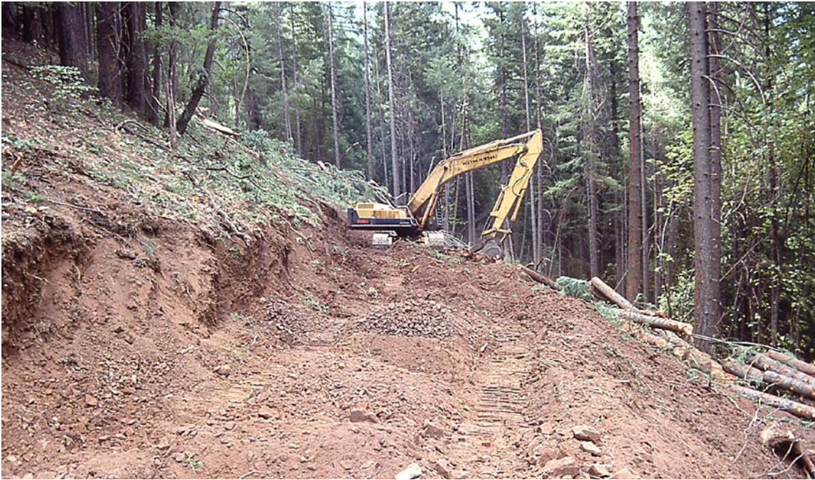
FIGURE 131. Excavators can perform a simple three step process of clearing and grubbing, excavating and subgrade development during construction of a balanced bench road. Using an excavator minimizes the volume of sidecast material. In the first pass an excavator operating from a pioneered bench removes logs and stumps, grubs the slope and installs a filter windrow of slash material at the base of the proposed fill slope. The second task is for the excavator to remove the overburden and place and compact the fill on the bench it has created (see piles of clean soil) and downslope above the windrowed slash. Thirdly, the uncovered, unweathered material is used to construct the bearing surface of the road.
