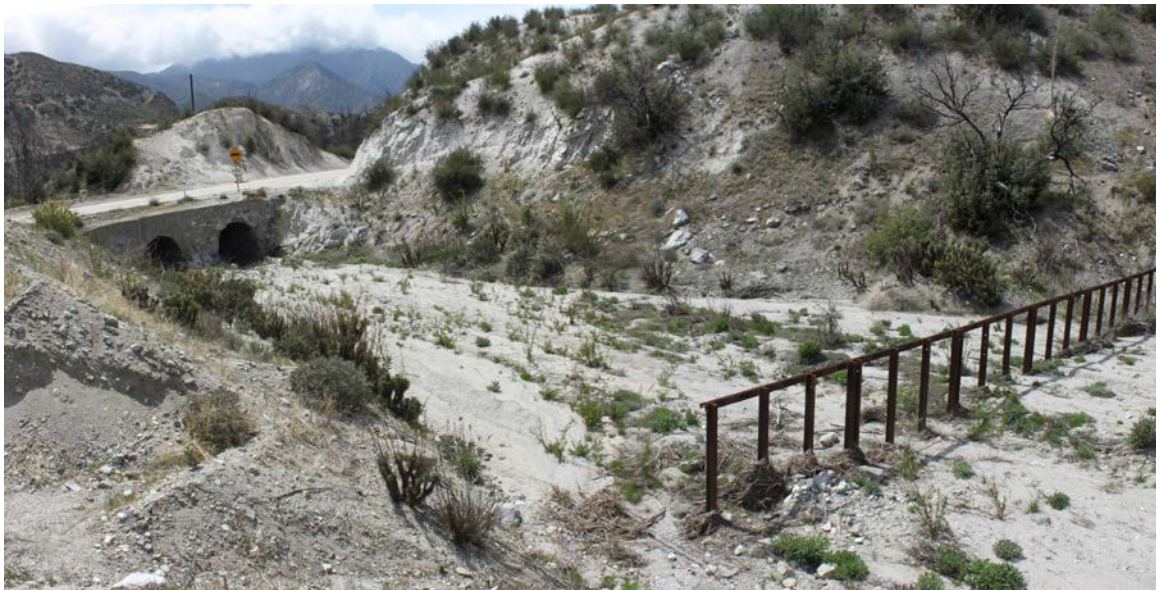
FIGURE 105. In larger streams, debris racks may need to be placed farther upstream from the culvert inlet. Limbs and branches floating down the channel are caught by the screen, but flow will back up and flood around the structure (as in this photo) if it is not extended into the bank. Debris racks or screens need regular maintenance to remove the accumulated debris. They should be made of durable metal posts and I-beams sized to resist the expected stresses and sunk deeply into the streambed for long term, secure installations.
