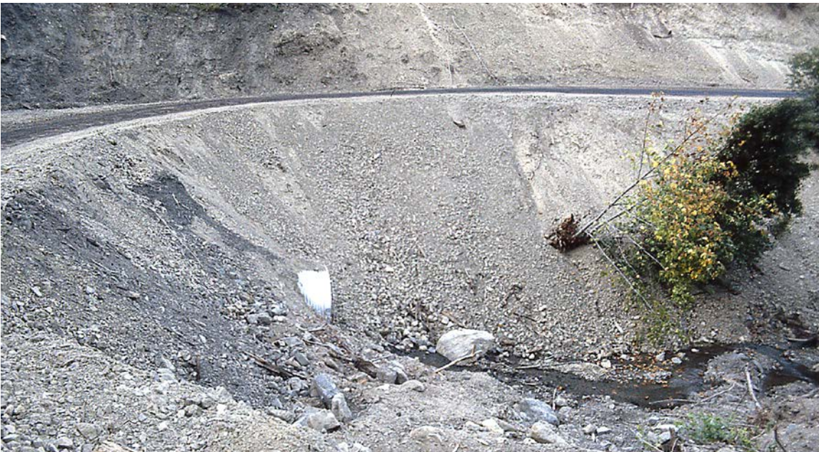
FIGURE 147. Uncontrolled sidecasting on the approach to this poorly constructed stream crossing delivers sediment directly to the stream channel. Roads built next to streams should be full bench endhailed, fill slopes should be at a stable angle (about 2:1), armor should be placed around the culvert, culverts should be extended approximately 6 feet beyond the base of the fill, and the slopes should be mulched and vegetated.
