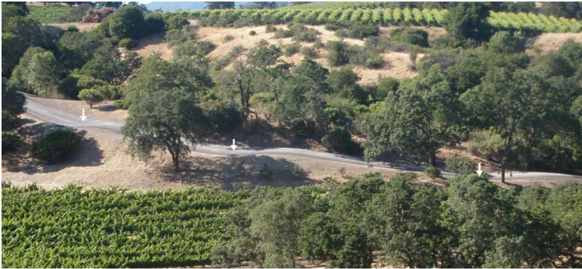
FIGURE 38. Rolling dips should be spaced on outsloped roads so that the road surface is well drained and free from erosion, and the slopes below each dip show minimal erosion. Three broad rolling dips (see arrows) are visible in this upgraded road reach used by both commercial and residential traffic.
