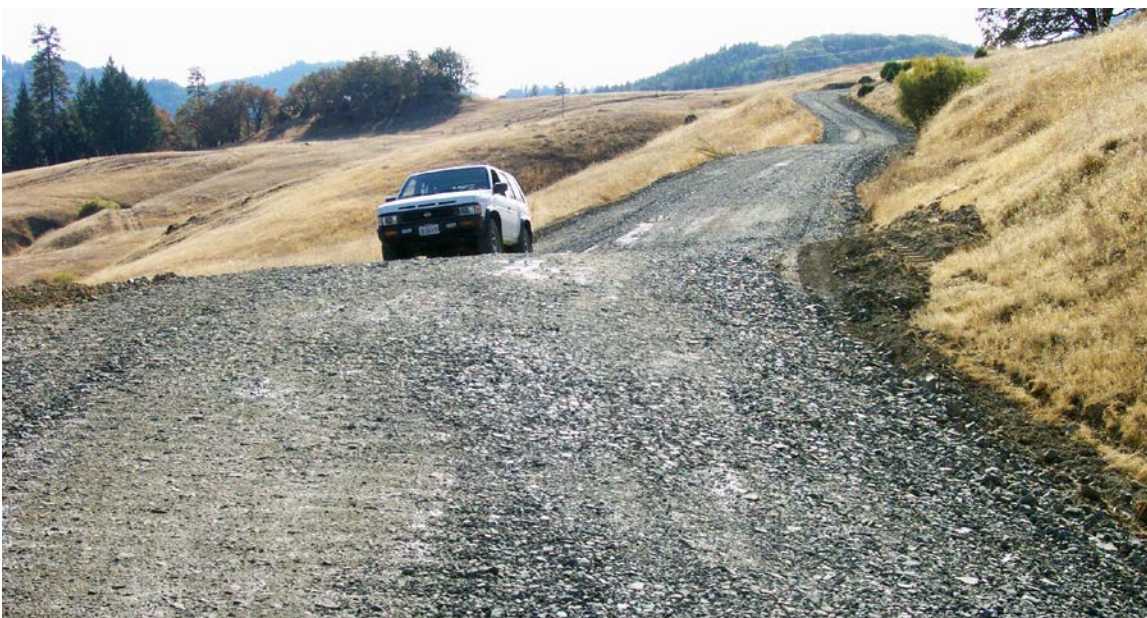
FIGURE 226B. The same road was converted to an outsloped shape, with broad rolling dips constructed at regular intervals, to disperse road runoff onto the adjacent grass covered slope and to disconnect road runoff from the nearby stream. Note that the ditch was filled and gravel was added to the low maintenance road surface.
