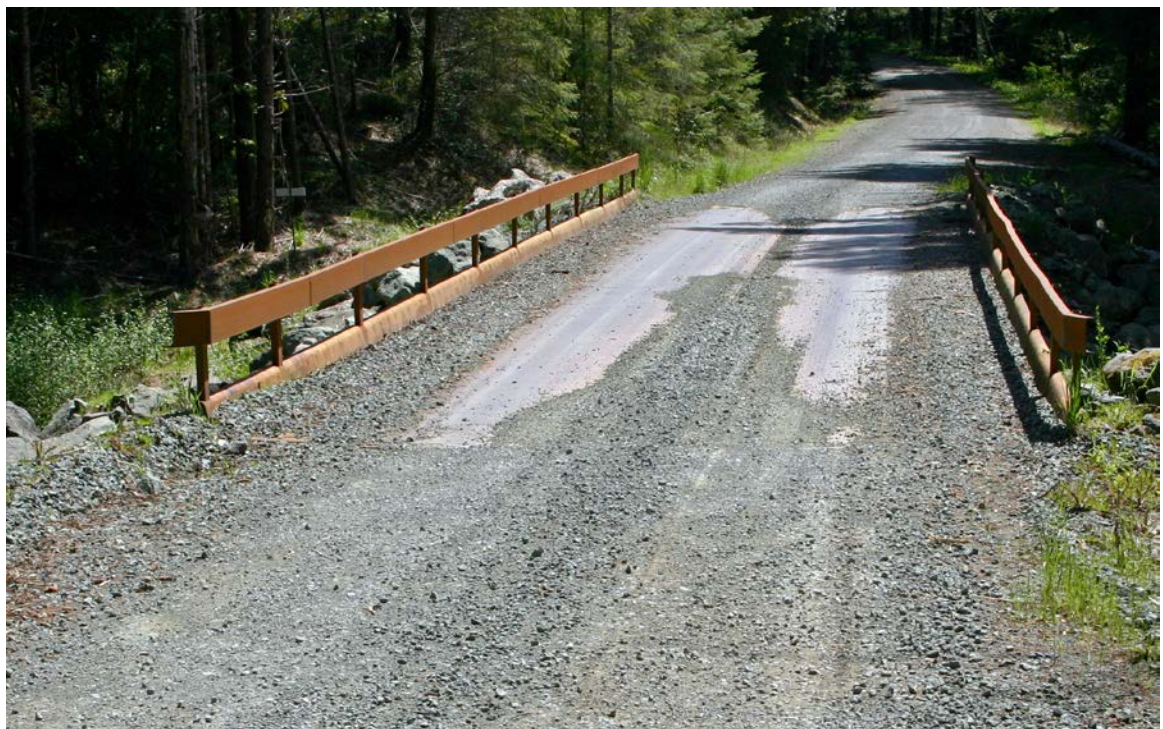
FIGURE 154. Wheel guards on a railroad flatcar bridge (see Figure 153) signal the driver that he is too close to the edge of the bridge. On this flatcar bridge, the road in the foreground slopes down to the bridge but the continuous steel wheel guard also seals the bridge surface so that all road runoff and sediment flows across the bridge and farther down the road before being dispersed onto the vegetated hillslope.
