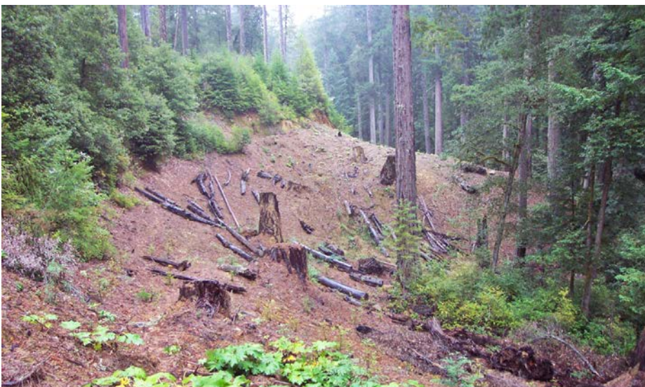
FIGURE 274B. After treatment, remnant stumps that had been buried by road construction and sidecasting were exhumed and gave the excavator operator a good idea where the original ground surface had been located. The outsloping was performed with little or no endhauling, as fill materials from the outside of the road prism were excavated, placed and compacted against the dry cutbank. Most of the cutbank has been buried and the slopes recontoured to their original form. The exposed soil was not seeded with grass, and rice straw was used as a mulch to prevent the introduction of non-native weeds. Litter from the adjacent forest quickly covered the surface.
