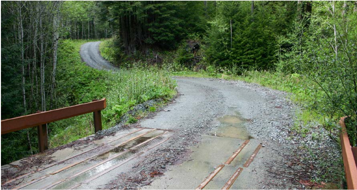
FIGURE 86. Rolling road grade is one method used to effectively drain a road and disconnect road runoff from streams. This road was dipped and then rises to the bridge crossing, ensuring that road runoff is drained off the road and onto the vegetated hillslope prior to reaching the crossing.
