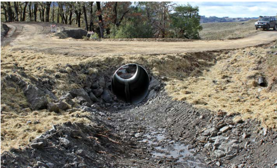
FIGURE 157A. Culvert installation in a shallow fill on a steep, boulder bedded Class II (non-fish bearing) stream replaced a severely undersized pipe (Figure 157a). The new six foot diameter culvert is set slightly into the original streambed and the inlet is armored to prevent erosion. The aggraded channel above the inlet (foreground) has been excavated and disturbed bare soil areas have been mulched and seeded. The roadbed dips into and out of the stream crossing with a critical dip placed just down-road of the left hinge line.
