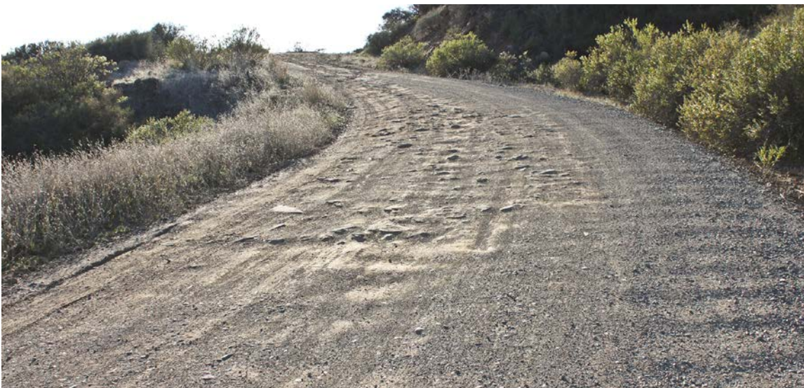
FIGURE 166. Road surfacing on this steep road reach has worn down the coarse base materials, making for a rough ride and reduced traction.
