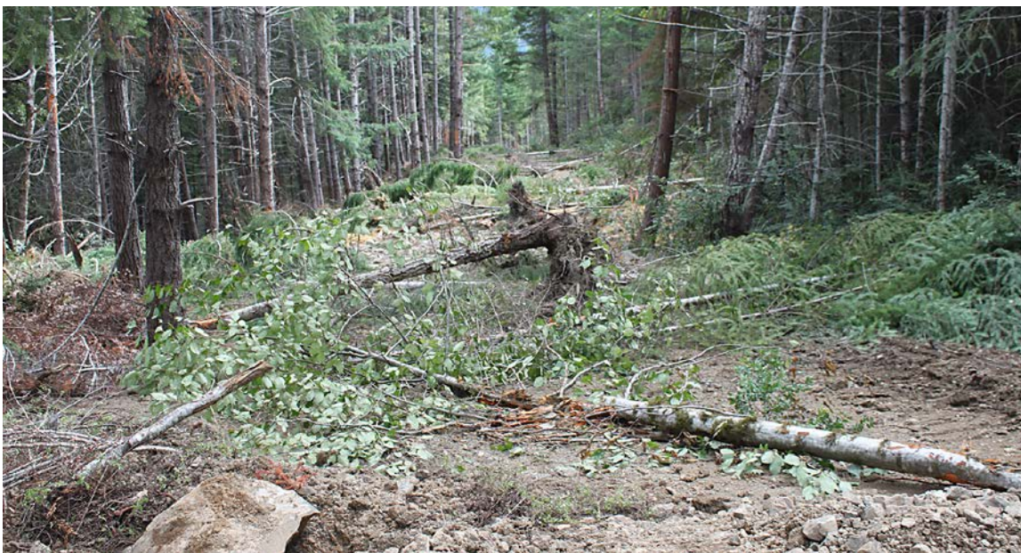
FIGURE 261. Decommissioned forest road in an area of gentle slopes and no stream crossings. Road decommissioning in “easy” terrain can be an inexpensive process that returns the former, compacted roadbed to productive forest or grasslands. Road decommissioning can be either permanent (never to be reopened) or temporary. The two treatments are generally similar and provide protection to the watershed for as long as the road is closed.
