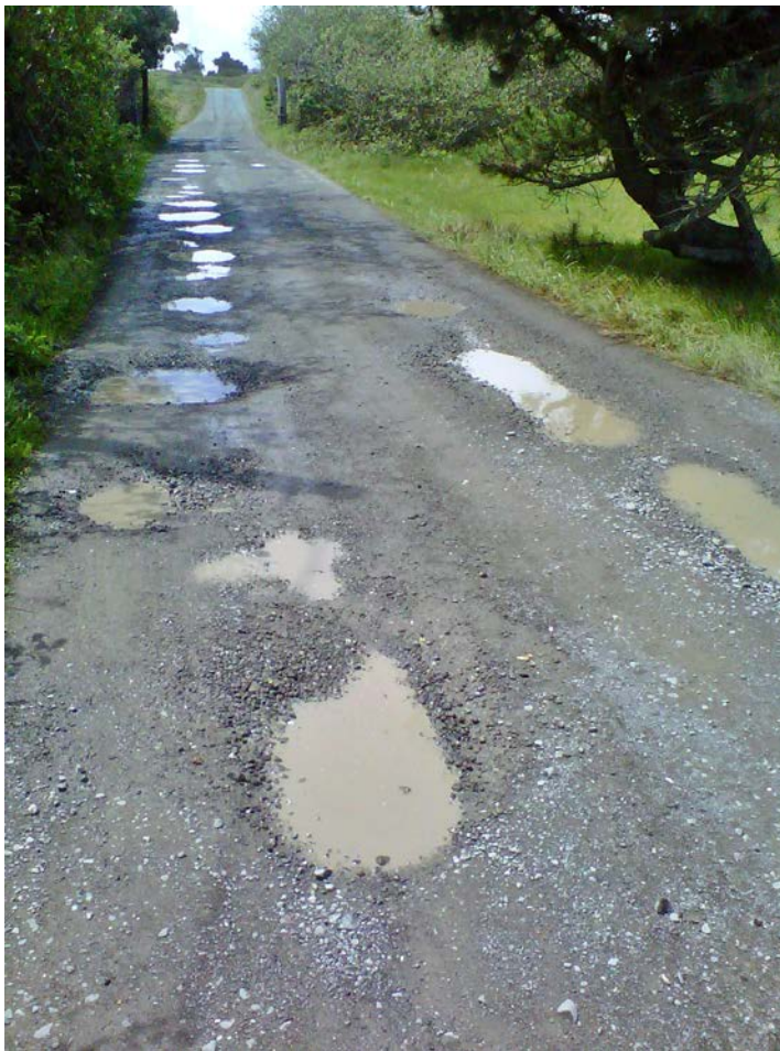
FIGURE 168. Standing water and the development of potholes are common indicators of poor road drainage.
