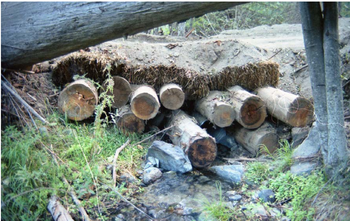
FIGURE 126. This small, temporary log crossing is constructed with a culvert at its base, with logs, straw bales and finally road surfacing material on top. A geotextile fabric can be used instead of straw to provide separation between the stream and the overlying road materials. Ideally, the road surfacing materials should be clean road rock or gravel (not dirt) that will not adversely affect water quality if some makes its way into the stream. Temporary crossings should be removed before each wet weather season.
