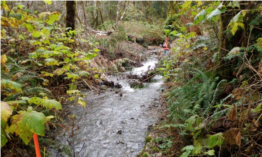
FIGURE 267B. The stream crossing fill was excavated and pushed down the alignment, away from the crossing. The gentle, excavated sideslopes were seeded, mulched with straw and covered with locally derived tree limbs and brush. The channel was excavated to the original streambed elevation, where rounded cobbles were exhumed, and constructed with the same width as the upstream and downstream channel reaches.
