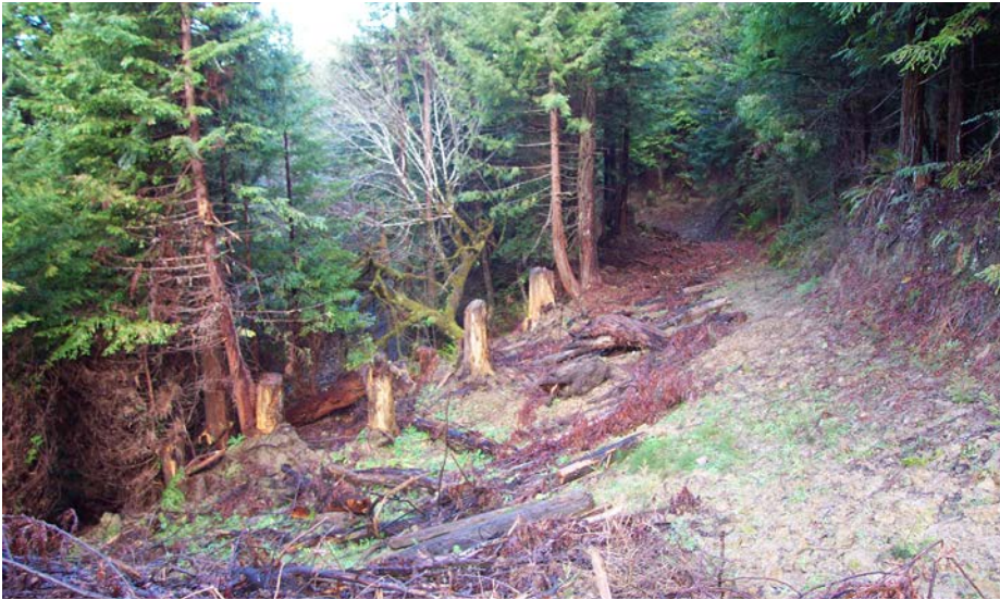
FIGURE 269C. The fill slope has been excavated and the spoil endhauled to a nearby spoil disposal site (exported outslope: EOS). Note the buried stumps that were exhumed and the basal flair that told the excavator operator where the original ground surface was located and how deep to dig. The cutbank has not been buried so the resulting outslope of the former road bench is strictly a result of roadbed and fill slope excavation.
