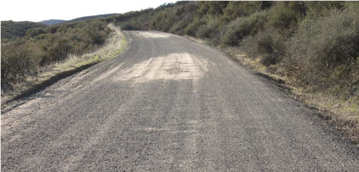
FIGURE 165. Because of traffic and erosion, road surfacing has locally worn down to the lighter color, finer grained native base materials beneath. The road needs resurfacing.
