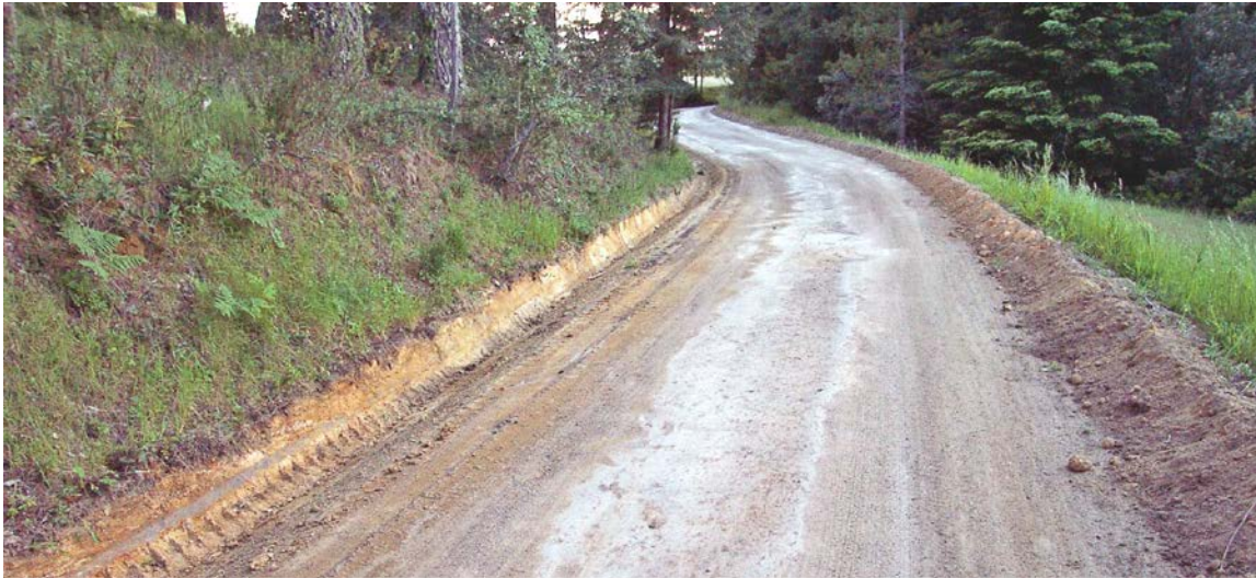
FIGURE 41. This outside berm on a crowned road prevents road surface runoff from draining onto the adjacent hillslope. If the road was insloped, the berm would not interfere with road drainage.
