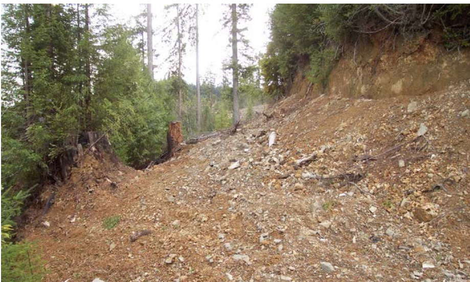
FIGURE 270B. Spoil excavated from the nearby unstable fill slope was hauled to this section of road and placed (and compacted) against the cutbank. This type of treatment is called an “Import Outslope” (IOS), where most of the fill used to outslope the former roadbed was imported from another, nearby excavation site. Using local spoil disposal sites, provided they are suitable, can save significantly on endhauling costs.
