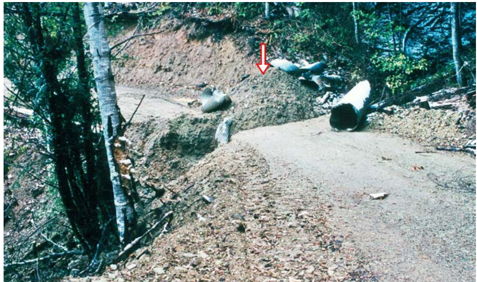
FIGURE 264. Poorly “decommissioned” stream crossing where the culvert was removed by trenching and the excavated spoil was piled next to the trench (see arrow) where it could easily erode into the stream. The entire stream crossing fill will be rapidly eroded and delivered to the stream if correct excavation and decommissioning treatments are not implemented before the next runoff event.
