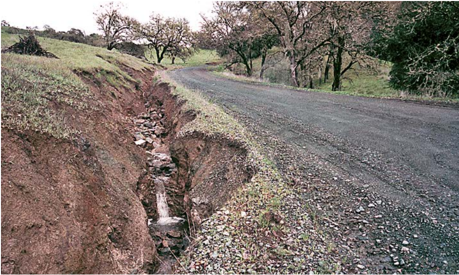
FIGURE 246A. Scoured roadside ditch carried runoff from the adjacent hillslope and from long lengths of the insloped road. The ditch gullied down to hard bedrock and discharged its runoff and eroded sediment to a stream just down the road.
