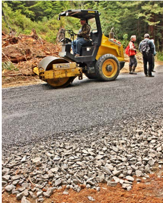
FIGURE 170. Road structural cross section showing a gravel surface course bound by finer material, overlying an angular base course spread and compacted on a stable, natural subgrade.
