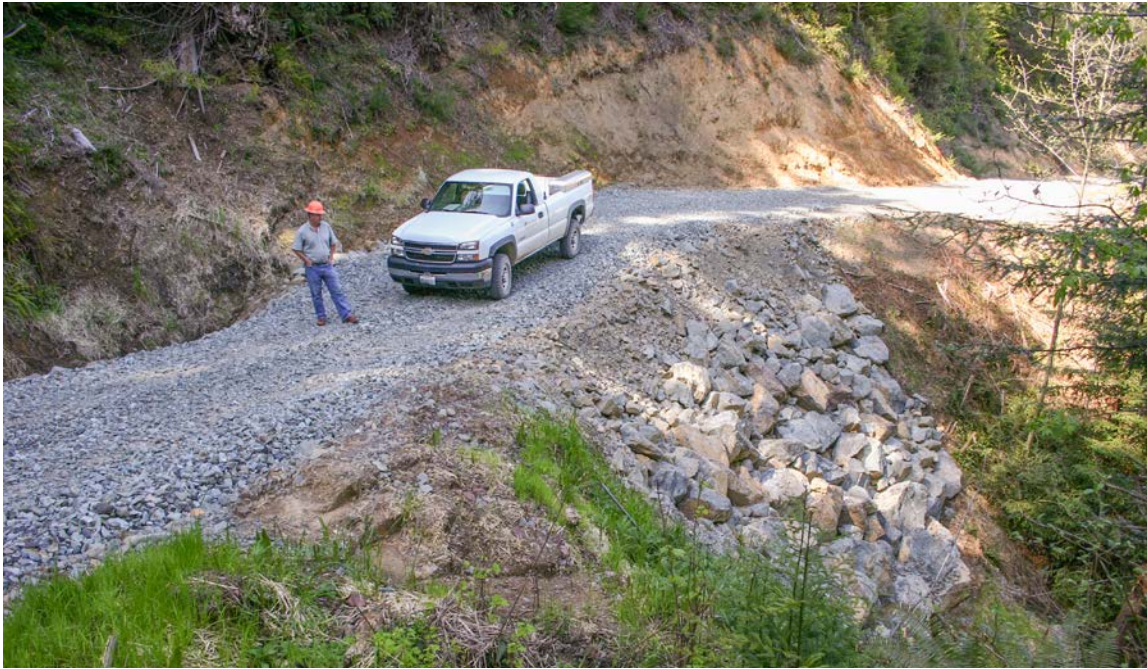
FIGURE 77. Road crossings of steep stream channels require fill slopes that often exceed a 2:1 slope gradient. This steep fill slope was stabilized with coarse rock armor embedded in a basal keyway.
