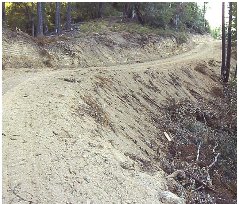
FIGURE 130. Road constructed by cutting and sidecasting (cut-and-fill road) in an upper hillslope location. A row of slash and organic debris along the base of the sidecast slope can help catch and filter soil eroded from the loose fill slope. Soil should only be sidecast onto gentle or moderate slopes that have been cleared and grubbed of vegetation, and where material cannot be eroded and delivered to a stream.
