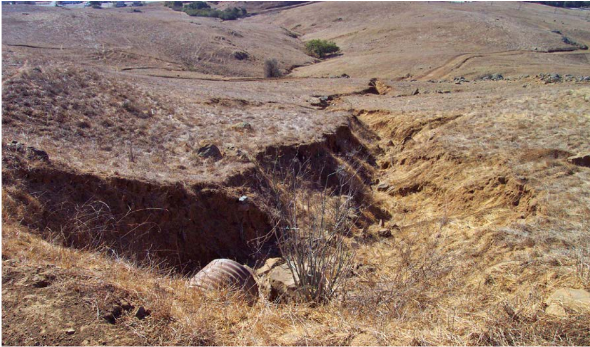
FIGURE 45. If ditches show excessive erosion, or long gullies form below the outlet of a ditch relief culvert, then the ditch is carrying too much flow and additional ditch relief culverts are needed up the road to break up the flow. Gullies below culvert outlets are a common source of hydrologic connectivity, delivering road runoff and eroded sediment to the downslope stream channel.
