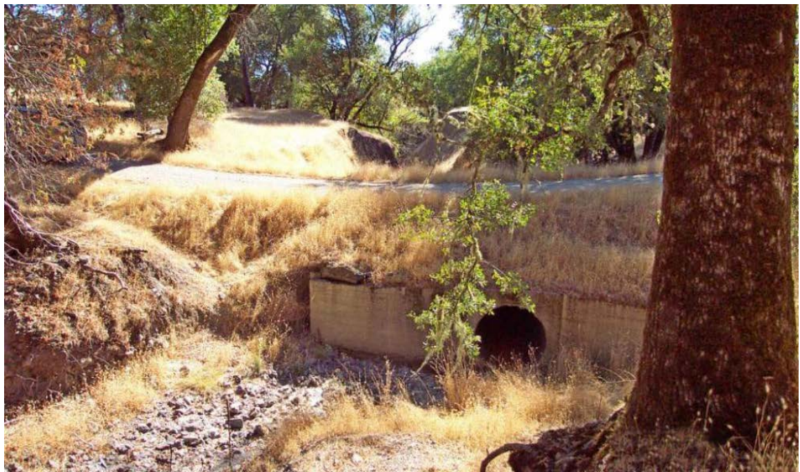
FIGURE 111. This concrete vertical headwall was installed on a ranch road stream crossing. The headwall increases culvert efficiency compared to a projecting barrel inlet, but is still prone to plugging by floating organic debris.
