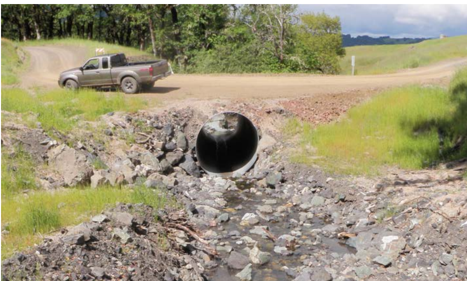
FIGURE 157B. After the first wet season (Figure 157b) the channel bed has self-armed and established a stable cross section leading to the inlet. Bare soil areas are covered with grass.
