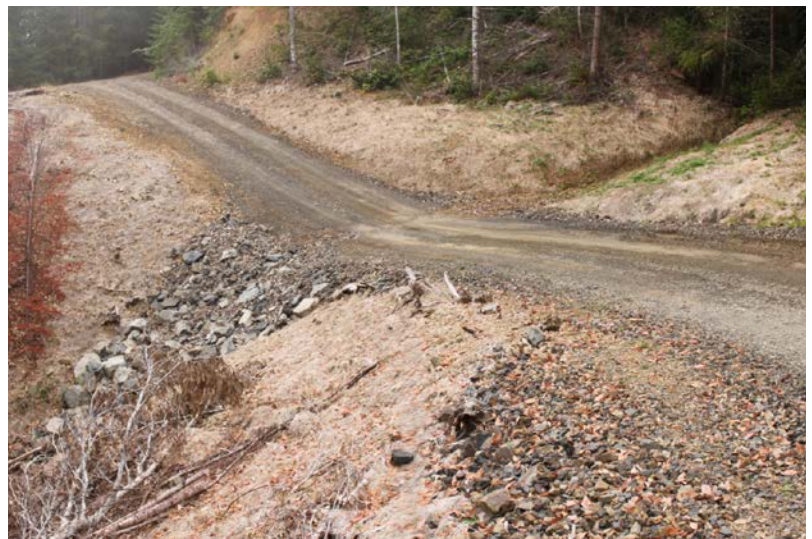
FIGURE 120. This armored fill crossing of a steep, ephemeral stream was constructed to provide a low maintenance crossing. The crossing has been deeply dipped to reduce the volume of road fill and to eliminate the potential for stream diversion. The fill slope has been heavily armored through the axis of the crossing to contain flood flows and prevent down-cutting. Armored fills cannot be used on fish bearing streams.
