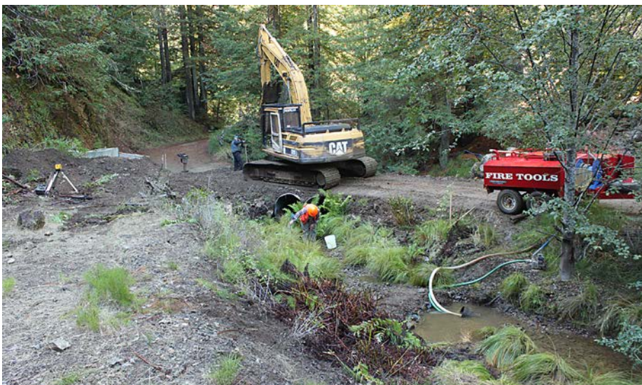
FIGURE 199. For larger streams, pump trucks, large pumps or multiple small pumps can be used to pump streamflow around project work sites. Here, a pump truck is used to temporarily divert flow in a fish bearing stream where dual culverts are being replaced with a railcar bridge. Young fish were removed from this fish bearing stream before project work started.
