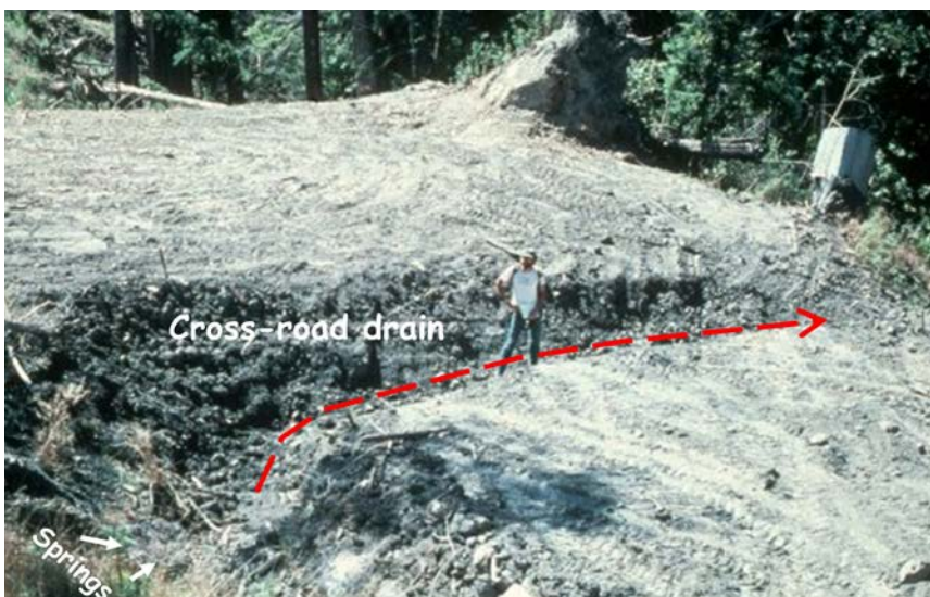
FIGURE 282. Deep cross road drains are constructed everywhere there is a spring or seep on the former road cutbank. This helps drain the road and the hillslope as uniformly and frequently as possible. Except for very short sections next to a cross road drain, inside ditches should not be retained.
