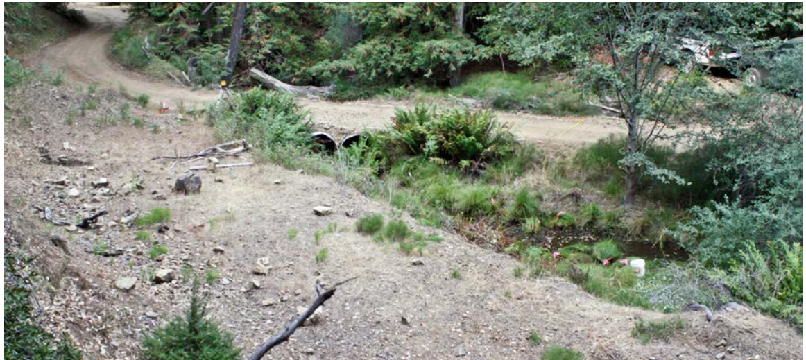
FIGURE 218A. Dual, undersized culverts were a partial barrier to fish migration on this rural road.
