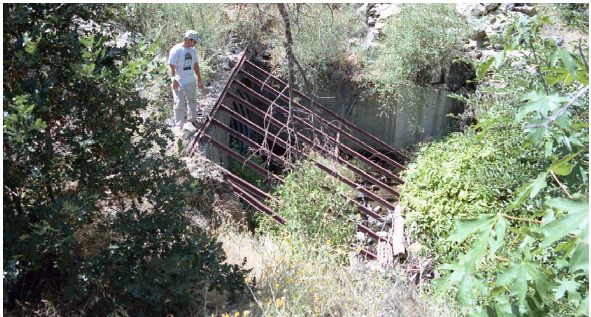
FIGURE 99. This 6-foot diameter culvert with concrete head- and wing-walls has a trash screen built over the inlet to catch floating debris. The design is flawed because it screens and catches small woody debris that would otherwise easily pass through the culvert. During a flood event, debris will quickly cover the trash screen and effectively plug the drainage structure. Screen bars should be more widely spaced and the trash rack should be installed in the stream channel somewhere upstream of the culvert inlet.
