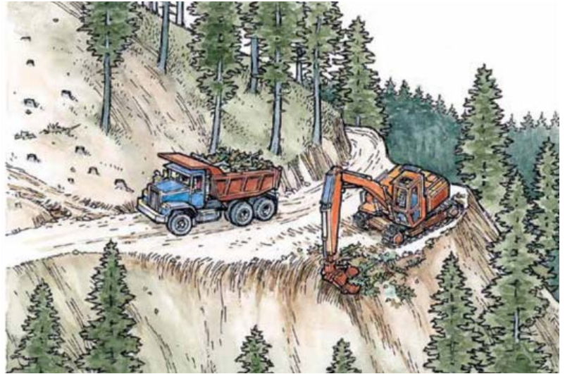
FIGURE 211. Unstable landing fill excavation. Oversteepened fill is removed from the landing edge and endhailed off-site to a stable location (Adams and Storm, 2011).
