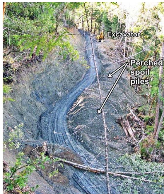
FIGURE 203. Sidecast constructed road built on a very steep inner gorge slope where a road should not have been built. Bulldozer constructed road perched large volumes of erodible spoil on the slope and debris slides have already delivered landslide debris to the stream channel below. This road is poorly located and upgrading will not reduce the failure potential. It is scheduled for permanent closure and the excavator (top of photo) is ready to begin decommissioning work.
