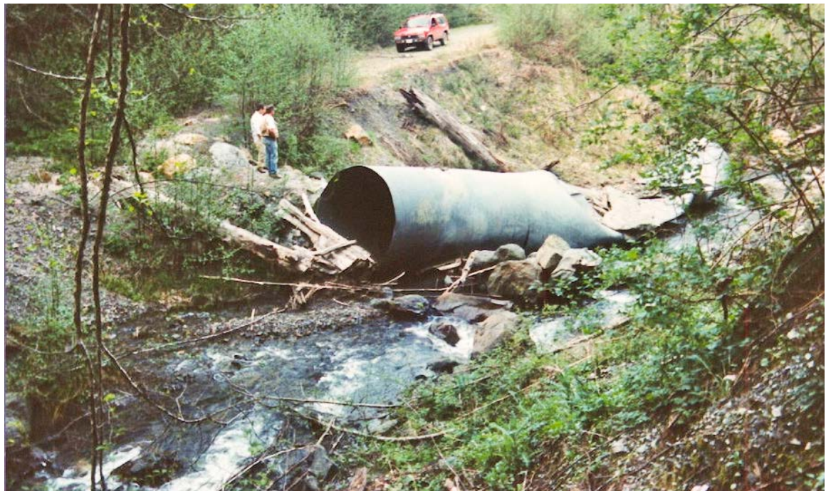
FIGURE 205. Under-designed or unmaintained stream crossings on older roads are prone to failure during large storms. This 8 foot diameter culvert was partially plugged (note wood at entrance) and flood flows overtopped and washed out the fill. During road reconstruction, stream crossings should be redesigned as temporary (and then removed) or upgraded for the 100-year flood flow, including passage of debris and sediment loads. When reconstructed, this crossing would either be fitted with an upstream debris screen or debris deflector, or a bridge would be installed.
