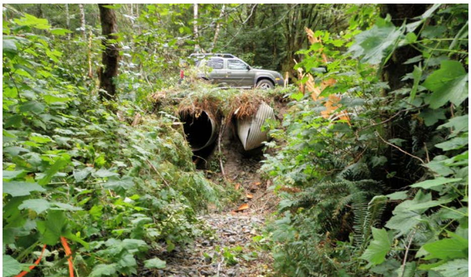
FIGURE 267A. Dual, undersized, elevated culverts at this small stream crossing have been a barrier to fish passage since the road was built decades ago. The outlet of the culvert on the right has been crushed closed, probably by heavy equipment performing maintenance work. Road and stream crossing decommissioning was used to permanently reopen the channel to fish passage.
