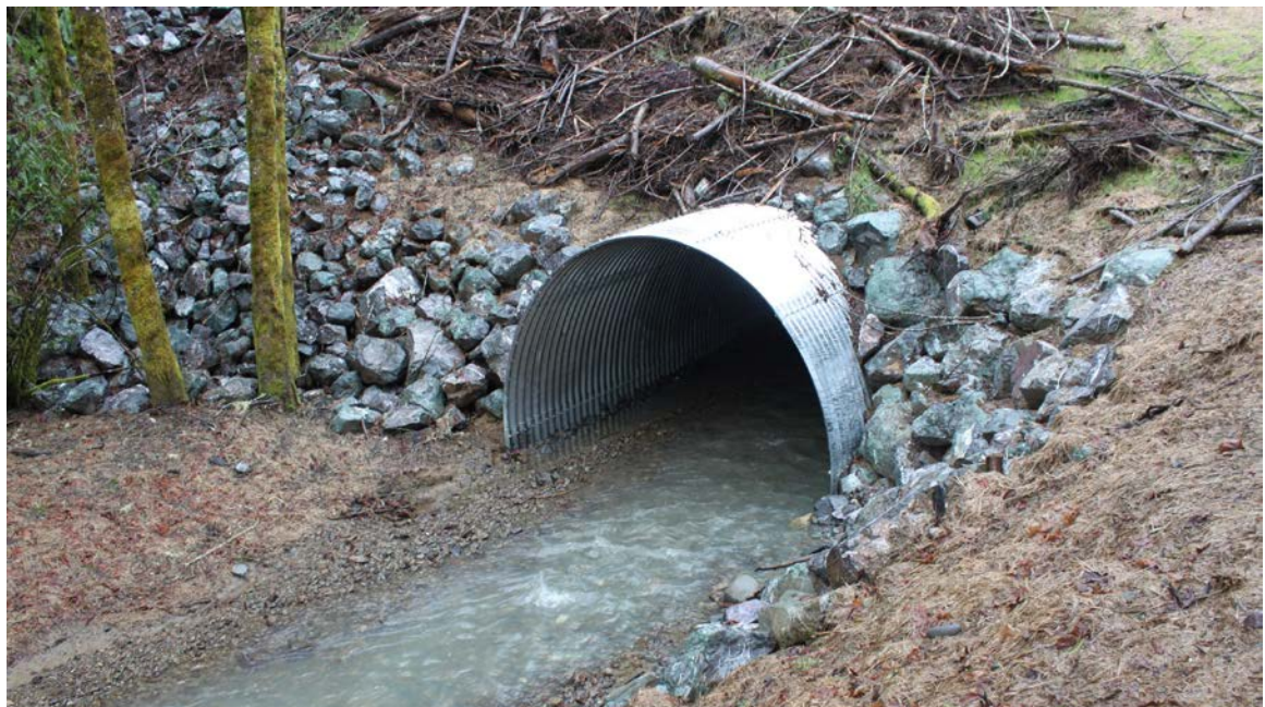
FIGURE 73. Embedded culverts are another type of stream crossing structure that allows continuous fish passage. This 10-foot diameter embedded culvert has a natural gravel and cobble streambed. It was installed to replace a small diameter culvert that was a barrier to fish migration.
