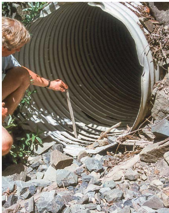
FIGURE 88. Abrasive bedload transport has worn through this aluminum culvert invert.
