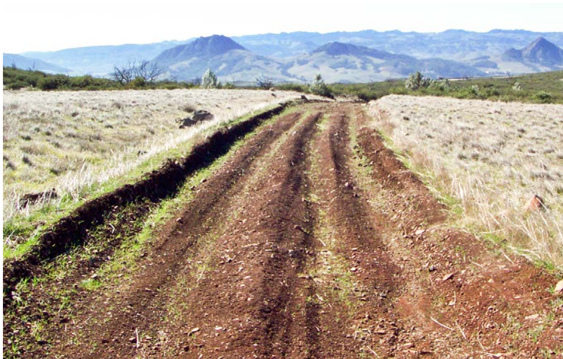
FIGURE 169. Road ruts on this seasonal road indicate a deteriorating subgrade that will either require traffic to be excluded during all but the driest periods, or strengthening with the application of a geotextile, base course, and surfacing materials.
