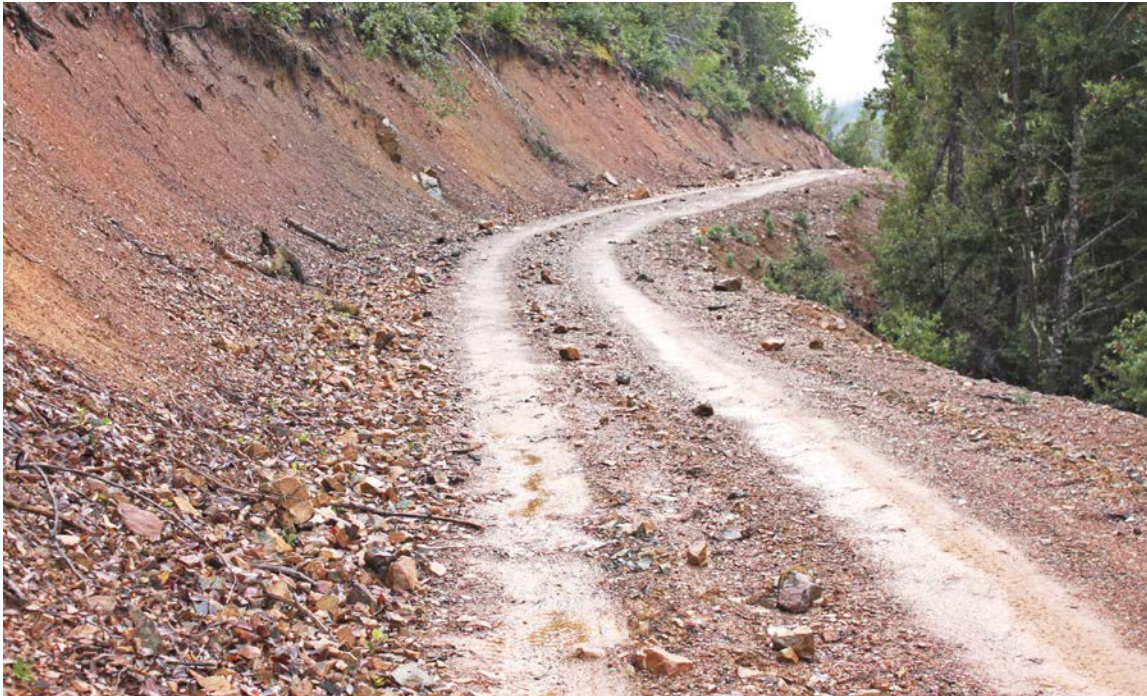
FIGURE 23. Full bench road. The height of the cut-bank, the slope of the natural hillside and the small amount of sidecast indicates that this road is full bench and cut entirely into native hillslope materials. Note that the road has no inboard ditch.
