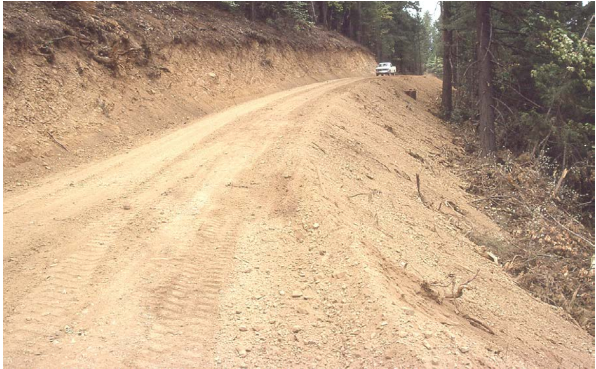
FIGURE 24. In contrast to the road in Figure 23, this partial bench road was built by extensive side-casting. At least half the roadbed is built on fill materials.
