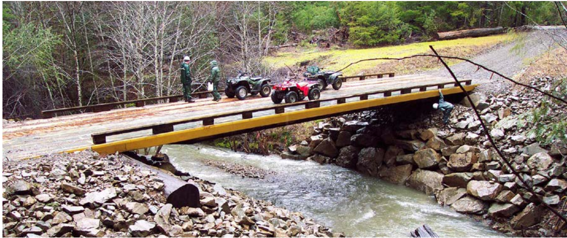
FIGURE 116. Low cost railroad flatcar bridges can be used for temporary crossings of incised stream channels, or they can serve as permanent water-course crossings. This 65-foot bridge spans the entire channel and was placed on large log abutments. The side-slopes have been protected with heavy rock riprap, and the natural channel width has been maintained through the crossing.
