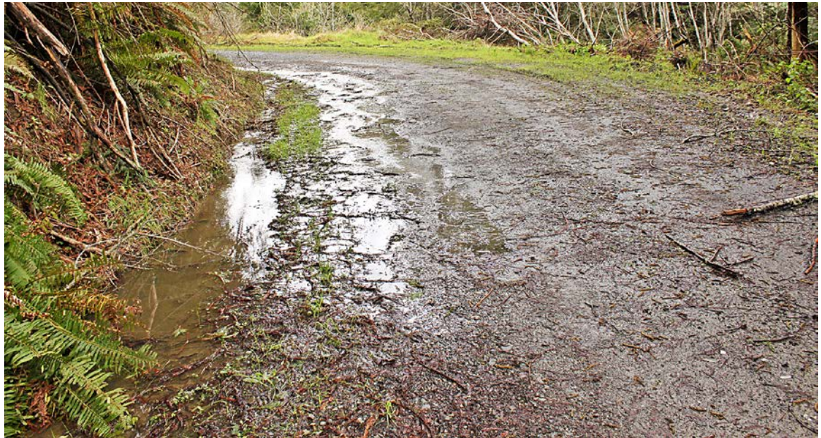
FIGURE 245. Over time, the ditch on this insloped road has filled with sediment. Road surface runoff now runs out of the ditch and onto the road surface, causing saturation and weakening of the road's structural section. Maintenance grading or excavation is needed to reestablish and deepen the ditch, thereby removing water from the road surface, draining moisture from the road base and surface materials, and re-strengthening the roadbed.
