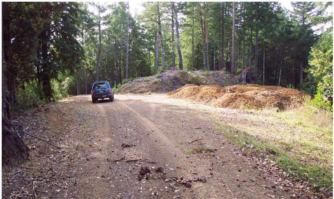
FIGURE 141. Typical spoil disposal site for endhauled spoil materials from a full bench road construction site. Spoil disposal site is located on a broad, gently sloping, dry ridge. Material is dumped, and will later be spread, compacted (by bulldozer) and seeded, mulched, and planted. Spoil material should be placed where eroded soil will not contaminate the road or ditch, or be delivered to a stream.
