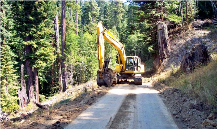
FIGURE 277A. Former private forest road, now in a U.S. BLM Biological Reserve, has been scheduled for out-sloping and conversion to a trail. The purpose of the decommissioning project was to recontour the old logging road and convert the route to hiking access for visitors and researchers. Note the stump in the right foreground.
