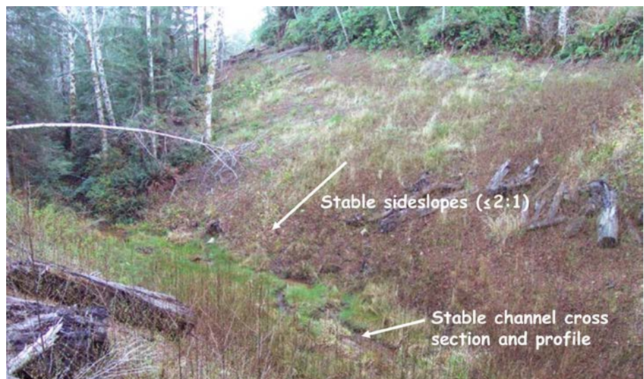
FIGURE 265. Properly decommissioned stream crossing, with 2:1 (stable) sideslopes, adequate channel width for flood flows, and a uniform channel grade (no humps of unexcavated fill) extending between the natural channel above and below the crossing. Because the slopes were dry, excavated spoil material was used to outlope the adjacent road approaches. The sideslopes were seeded with grass and straw mulched to minimize erosion following decommissioning.
