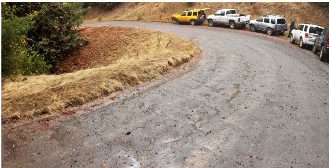
FIGURE 82. This newly upgraded stream crossing fill was protected from road runoff and erosion by the installation of a drainage berm along the road. Once the fill is vegetated and stabilized, the berm can be safely removed.
