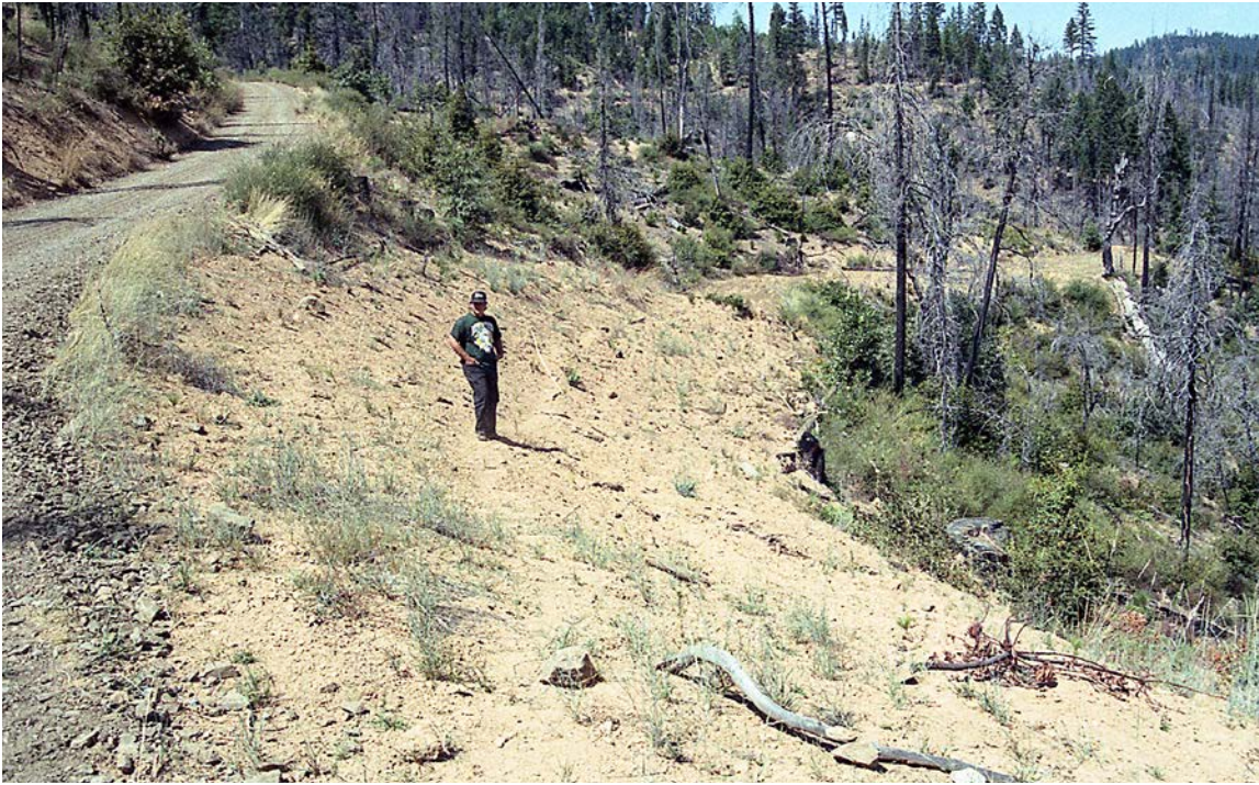
FIGURE 292. Severe outslipping, which prevents vehicle access, should only be used on temporary roads and decommissioned roads where all stream crossings have first been removed, unstable fill slopes have been excavated or stabilized, and road surface drainage is permanently dispersed. To help ensure vehicles do not use the closed road, logs, boulders and brush can be spread over the surface, especially near the beginning of the road, to discourage unwanted traffic. These roads should need no future maintenance, so vehicle access is no longer needed.
