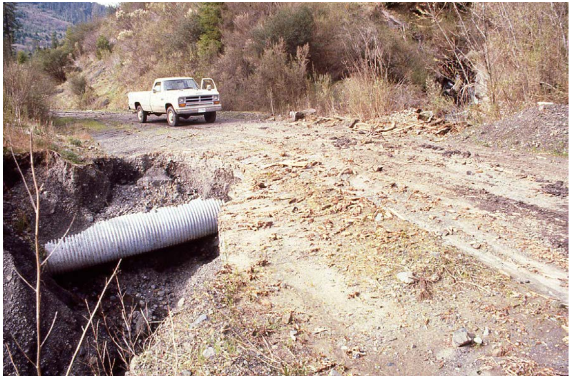
FIGURE 64. Eroding stream crossing after a single storm on an unmaintained road. The culvert plugged and flood flow overtopped the fill, initiating a head-cut. In addition to being undersized, the culvert was installed at a flat gradient that is more prone to inlet plugging with debris. If left uncorrected, the crossing fill would continue to erode and deliver the eroded sediment downstream.
