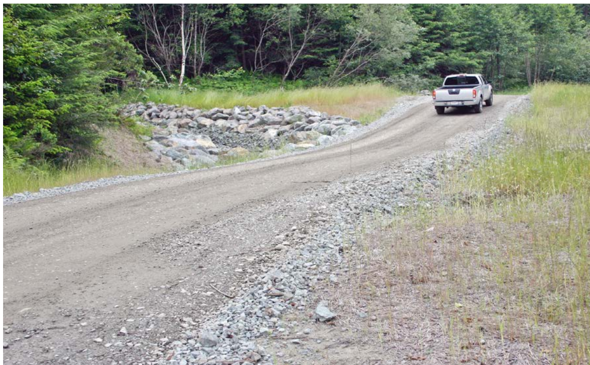
FIGURE 69. A gradually climbing road changes grade over the small stream crossing, thereby eliminating the possibility for future stream diversion. The dip is broad and gentle to accommodate all traffic, and designed to carry peak flood flows across the road and back into the channel with minimal erosion and sediment delivery.
