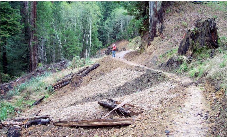
FIGURE 277B. The former road was decommissioned by excavating the sidecast fillslopes and placing the excavated fill against the dry cut banks. The excavated fillslopes were covered with rice straw and woody debris to control erosion while preventing the introduction of exotic grass and weed species. The once-straight road has been converted into a winding trail that follows the original landscape contours. Topographic swales and stream channels have all be excavated and recontoured
