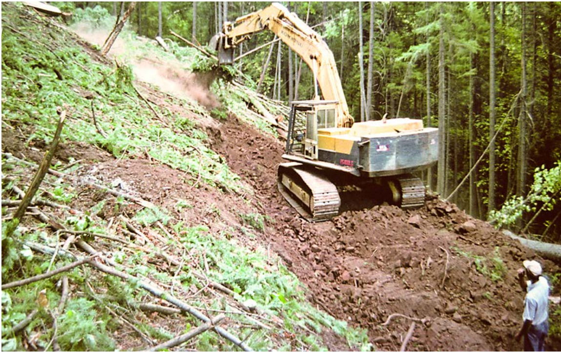
FIGURE 129. Hydraulic excavators have become the preferred piece of heavy earthmoving equipment for wildland road construction. Here an excavator is clearing and grubbing the alignment for a new forest road. All organic material must be removed from the alignment and woody debris should not be incorporated in fill materials.
