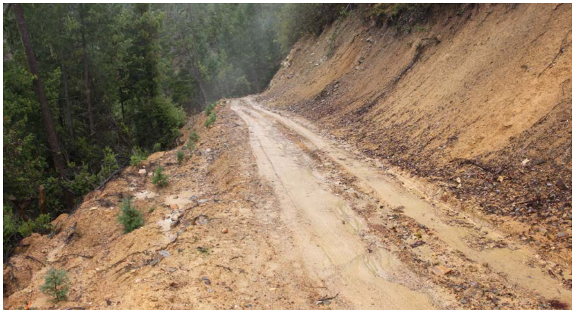
FIGURE 143. Sidecast road construction on steep inner gorge slopes above a fish-bearing stream. Fine grained sidecast materials are perched on 70% slopes and show signs of instability and pending failure. The remaining, stable part of the roadbed is on the road cut.
