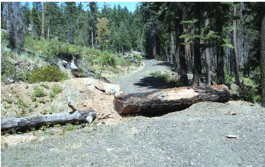
FIGURE 249B. If barricades or physical barriers are used, they must be removed with heavy equipment before maintenance activities can be performed. They should not be used on roads which have stream crossings since these need to be inspected and maintained during and following storms.
