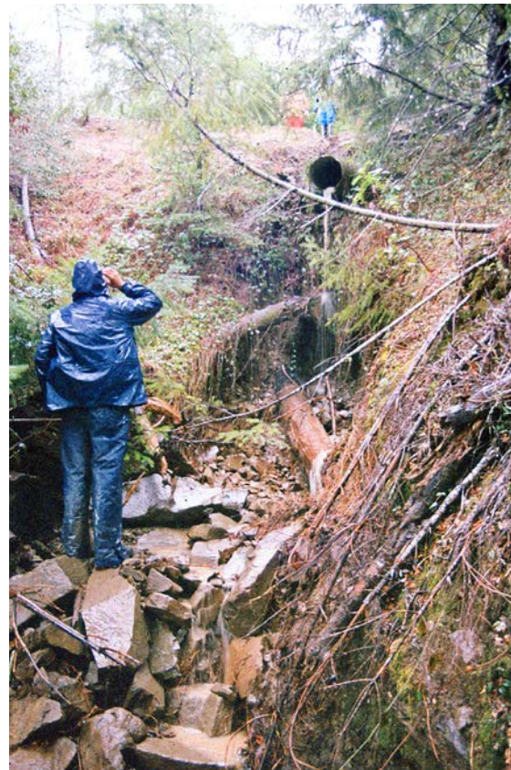
FIGURE 201. A road inventory crew surveys stream crossings and other under-designed elements of a road, identifying needed upgrades along the route. The most important things to identify, and upgrade, are those that could cause road or stream crossing failures (like this perched, undersized stream crossing culvert), or that deliver road runoff and fine sediment to the stream system.
