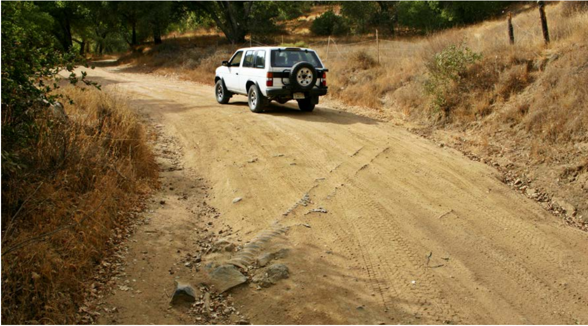
FIGURE 235. This road surface has worn down over years of use, grading and erosion to the point that a formerly buried ditch relief culvert has been exposed in the roadbed. When installed, the culvert was probably 2 or 3 feet below the road surface. Both gravel surfaced and unsurfaced (native) roads wear down over time, due to traffic and erosion. It is often not noticeable until the gravel is gone, the road becomes entrenched (through cut) or the top of cross drain culverts become exposed.
