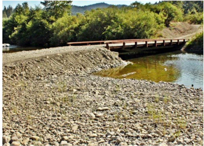
FIGURE 127B. A temporary bridge crossing should be used where migrating adult or juvenile fish need to pass beneath the crossing. This temporary bridge crossing spans the active summer channel and the abutment in the channel is composed entirely of clean stream gravels. All temporary low water crossings should be removed before the first seasonal rains.
