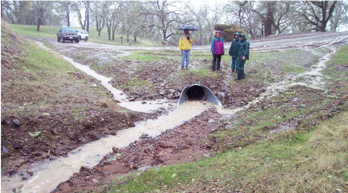
FIGURE 5. Hydrologic connectivity occurs where road and ditch runoff is delivered to the natural stream channel system. It most commonly occurs where road ditches discharge road runoff and eroded sediment directly to stream crossing culvert inlets. In this photo, both road ditches are hydrologically connected to the natural stream where it enters the culvert.
