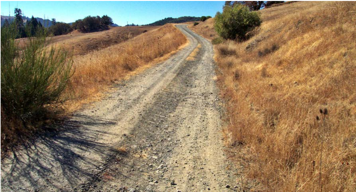
FIGURE 226A. Rural subdivision road was insloped and rutted prior to treatment. Runoff from the eroding roadbed was delivered directly to a stream channel.
