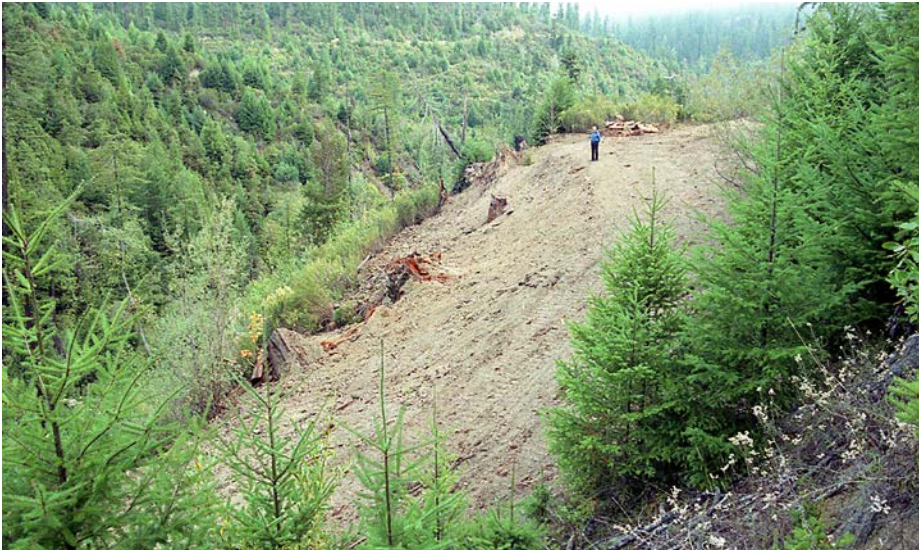
FIGURE 272B. The excavation required a temporary road be built across the middle of the long fill slope to reach all the unstable material. The concave excavation surface mimics the shape of a potential slide plane and thereby assures that most of the unstable fill material has been removed. Spoil materials were pushed up against the inside of the large landing, entirely on a stable, excavated bench. As in Figure 271B this type of out-sloping is called an “Inplace Outslope” (IPOS), where all the excavated materials were stored locally (note person for scale).
