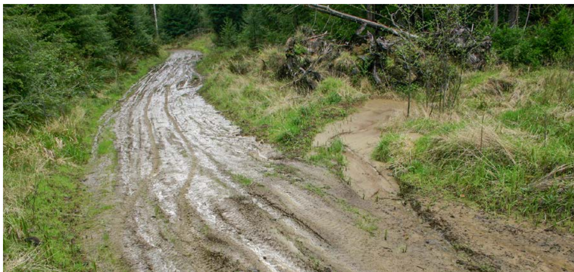
FIGURE 57. This seasonal road was built on fine grained soils that exhibited poor drainage and high rates of soil erosion. Even minor traffic during the wet season caused damage to the roadbed and rapid erosion clogged and filled ditches, waterbars and rolling dips.
